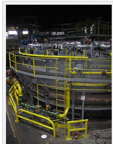
General Dynamics' Bliss Three Forge Furnace is a natural gas-fired rotary hearth furnace used to heat steel before forging. Refurbished with a new high performance refractory, high efficiency burner controls, and natural gas recuperators, the furnace improvements translated into a 25% reduction in natural gas consumption. Photo credit: General Dynamics.
