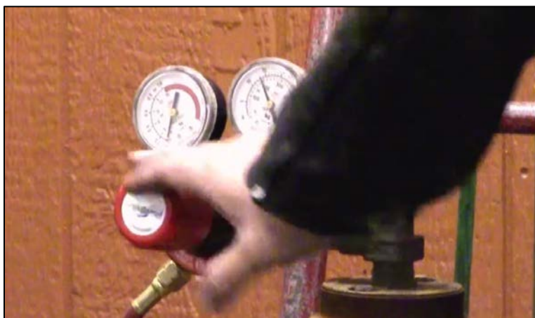
CAPTION 6. THE ADJUSTMENT SCREW ON THE ACETYLENE VALVE IS BEING SET TO 5 PSI.
