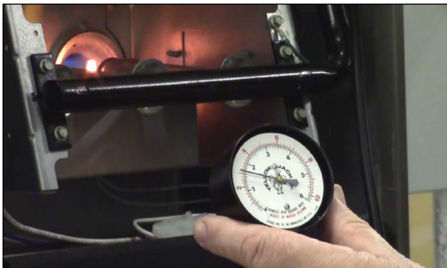
CAPTION 3. THE NEEDLE ON THE GAUGE MOVED WHEN THE GAS VALVE OPENED. IN THE PHOTO, THE PRESSURE IS AT 3 INCHES OF WATER COLUMN. THE MANUFACTURER'S RATING FOR GAS PRESSURE IS 3 ½ INCHES OF WATER COLUMN.
