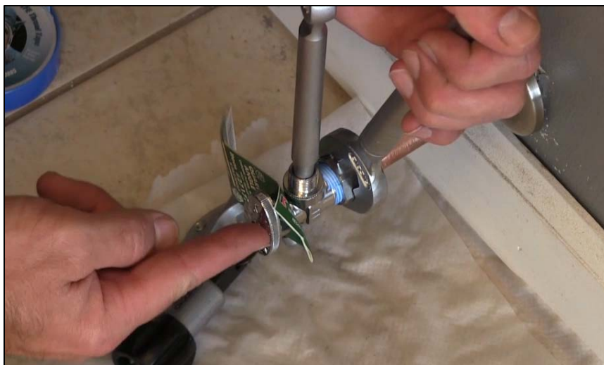
CAPTION 21. THE INSTRUCTOR POINTS AT THE FITTING, WITH A ONE-STOP WRENCH HOLDING IT IN PLACE, AND A CRESCENT WRENCH POSITIONED ON THE NUT.
