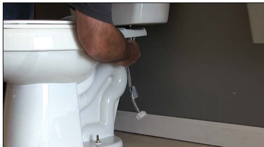
CAPTION 28. THE INSTRUCTOR TIGHTENS THE BOLTS ON THE TANK TO THE TOILET BOWL.
