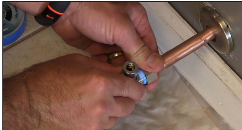
CAPTION 20. THE NUT IS TIGHTENED DOWN ONTO THE FITTING. THE FERRULE (NOT SEEN IN PHOTO) WILL WRAP AROUND THE PIPE AS THE NUT IS TIGHTENED DOWN.
