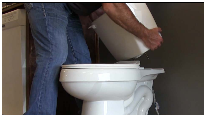
CAPTION 27. THE INSTRUCTOR SETS THE TOILET TANK ON THE INSTALLED TOILET BOWL.
