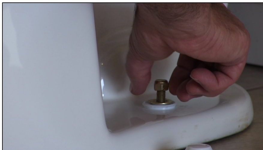
CAPTION 26. THE INSTRUCTOR STARTS INSTALLING THE BOLT ON ONE SIDE OF THE TOILET BOWL.
