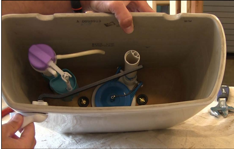
CAPTION 13. INSIDE VIEW OF THE FINISHED TOILET TANK, WITH THE FLUSH HANDLE ALREADY INSTALLED.
