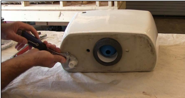
CAPTION 8. NUT FOR THE FILL VALVE IS TIGHTENED WITH A CRESCENT WRENCH.
