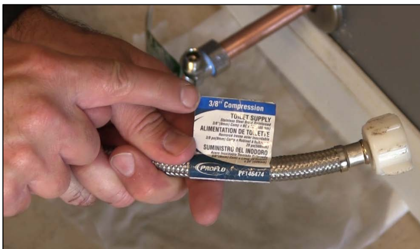
CAPTION 22. THE INSTRUCTOR SHOWS THE TYPE OF TOILET SUPPLY LINE HE WILL BE INSTALLING.
