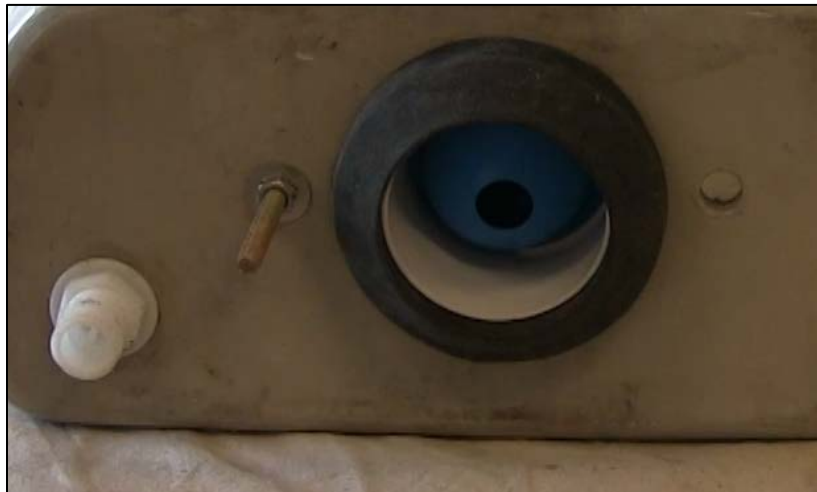
CAPTION 10. (FROM LEFT TO RIGHT) THE INSTALLED FILL VALVE, BOLT, AND FLUSH VALVE.
