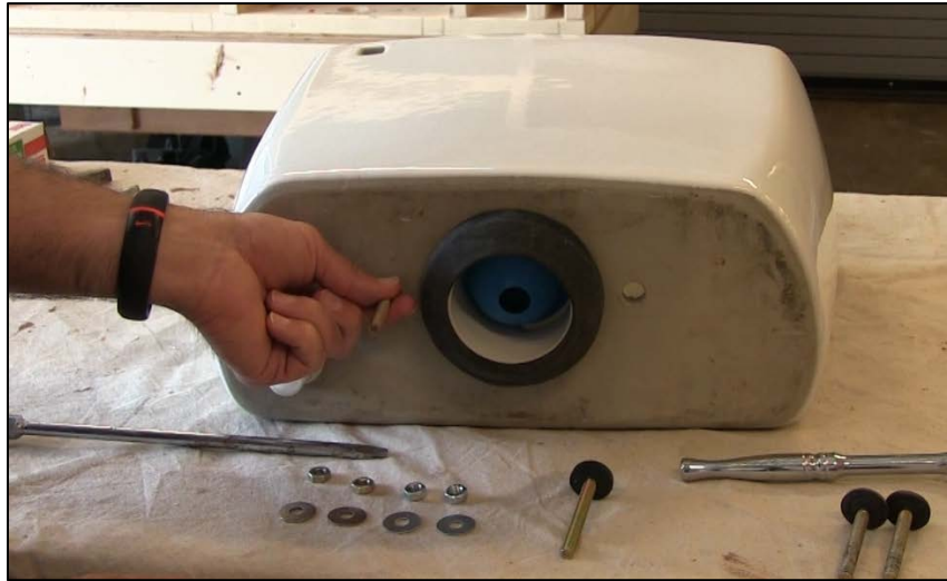
CAPTION 9. THE INSTRUCTOR INSTALLS ONE OF THE TWO BOLTS ON THE TANK.
