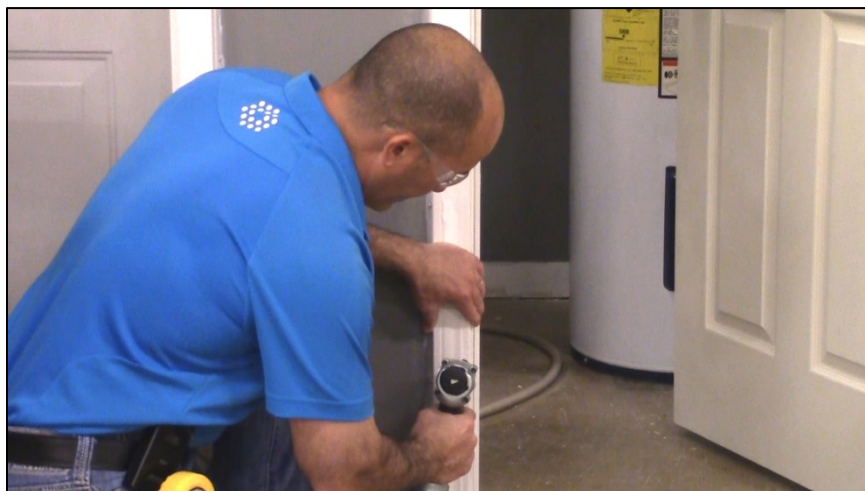
CAPTION 8. THE INSTRUCTOR NAILS THE CASING, STARTING FROM THE BOTTOM OF THE LATCH SIDE.
