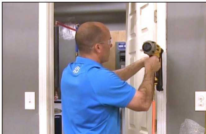
CAPTION 10. THE INSTRUCTOR USES A STRAIGHT FINISH NAILER TO FINISH INSTALLING THE CASING.
