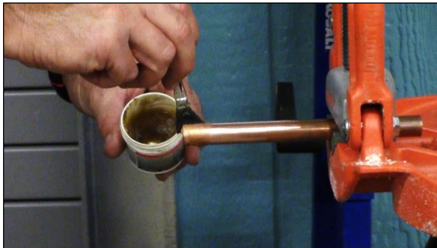
CAPTION 6. FLUX IS BRUSHED ONTO THE END OF THE PIPE WHERE THE FITTING WILL BE INSTALLED
