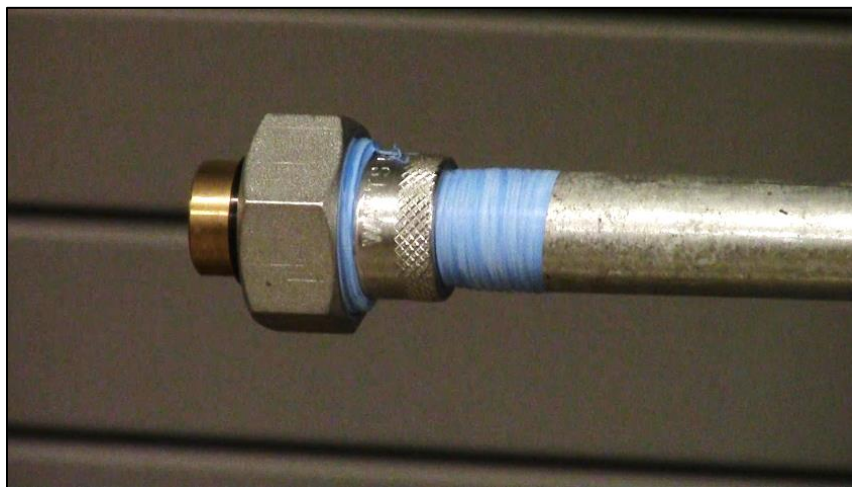
CAPTION 19. A CLOSE-UP OF THE HAND-TIGHTENED FITTING AROUND THE TEFLON-WRAPPED GALVANIZED PIPE.
