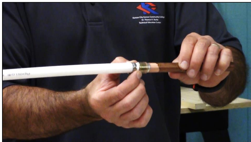
CAPTION 17. THE INSTRUCTOR HOLDS THE FINISHED PRODUCT: A SUPPLY LINE TRANSITIONING FROM COPPER TO PEX.
