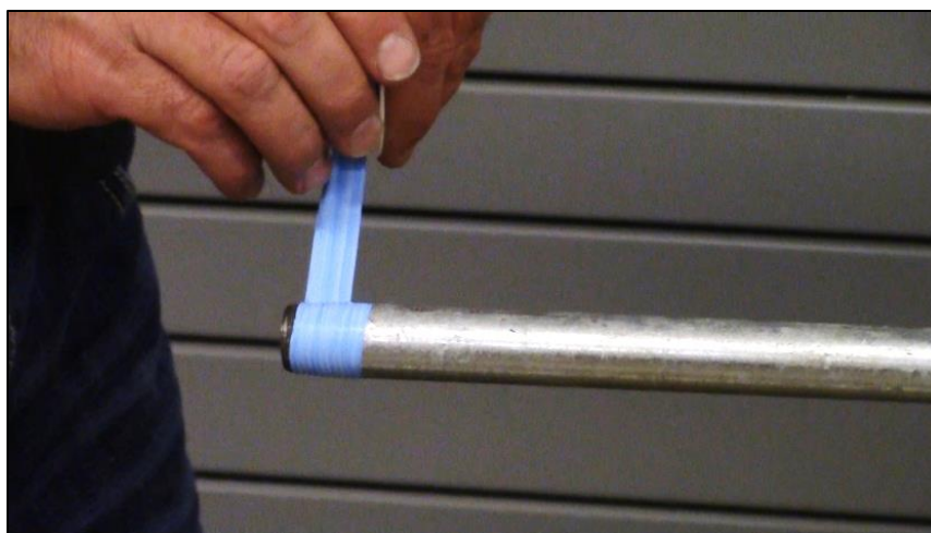
CAPTION 18. TEFLON TAPE IS WRAPPED AROUND THE THREADS OF THE GALVANIZED PIPE.
