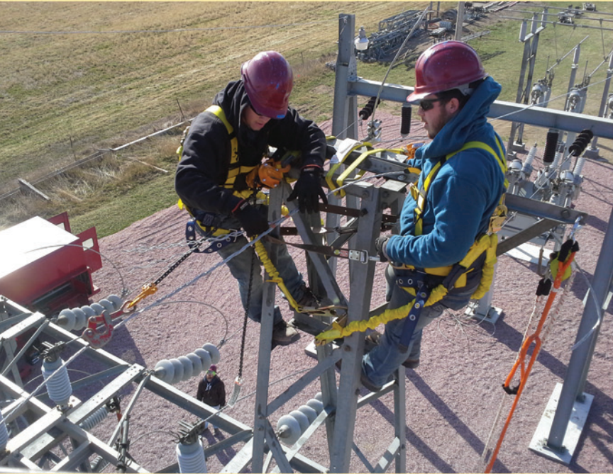
Mitchell Technical Institute Substation students install new equipment at the campus training field.
