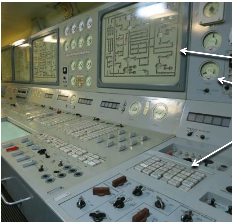
Fig. 15-4 This panel shows many discrete devices as well as mimic panels showing process lines.
