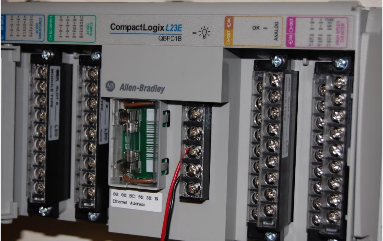
Fig. 3-19 View of CompactLogix L23E with Wiring Exposed
