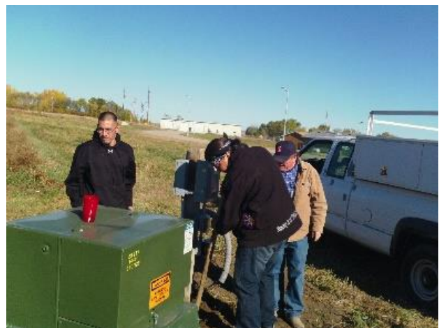
Students in SBC’s electrical program receive training on a local underground transformer. This work done in the field is paired with a new, grant-funded electrical lab to provide hands-on training.
