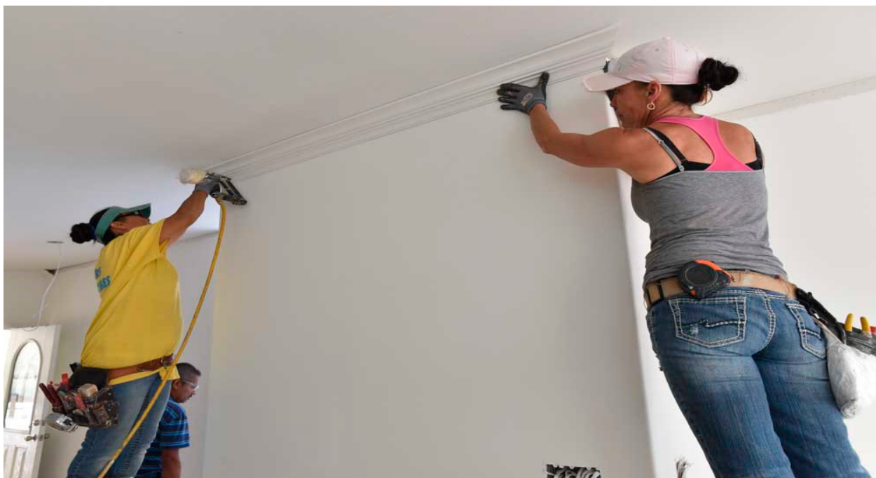
FIGURE 1.59, 1.60, & 1.61: TRIM WORK, REMAINING ELECTRICAL INSTALLMENT, AND OTHER FINISHES ARE DONE IN THIS STATION
