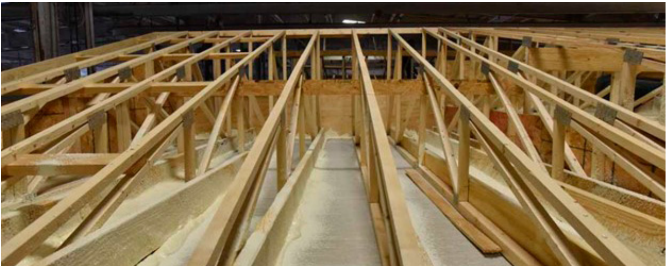
FIGURE 1.39, 1.40, AND 1.41: TRUSSES AND RAFTERS ARE SET VERTICALLY ON THE GYPSUM BOARD AND ATTACHED WITH ADHESIVE MATERIAL AND APPROPRIATE FASTENERS.
