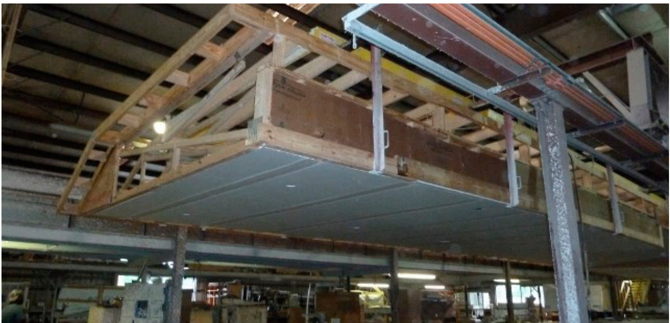
FIGURE 1.42: THE CEILING IS FINISHED AND THE ROOF IS READY TO BE INSTALLED AT THIS STATION.
