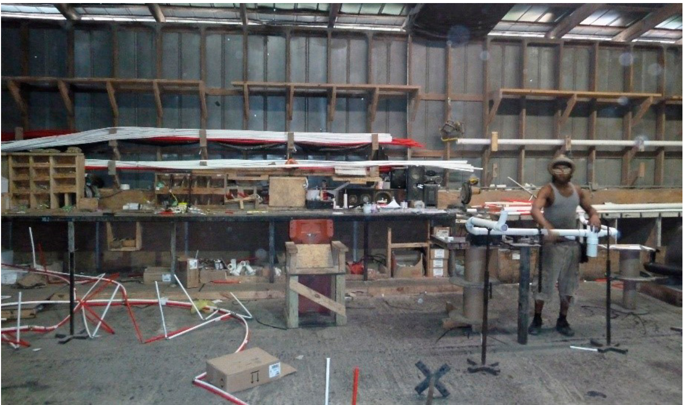
FIGURE 1.17: PARALLEL TO THE CHASSIS STATION AND THE FLOORING STATION, THE OFF-LINE PLUMBING STATION IS PREPARING THE PIPES THAT WILL BE INSTALLED IN THE FLOORING DEPARTMENT
