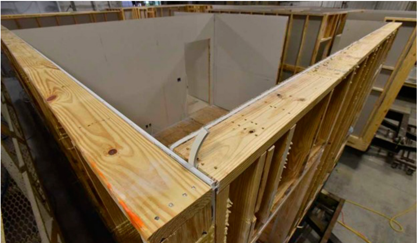
FIGURE 1.35: GASKETING MATERIAL IS USED TO AVOID AIR EXCHANGE IN BETWEEN DIFFERING WALL TYPES.
