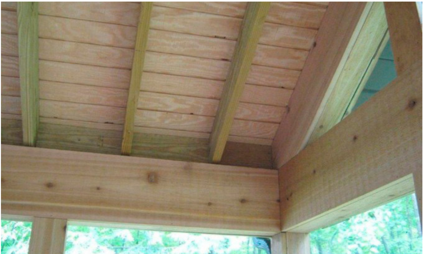
FIGURE 1.37: THE STRUCTURE SUPPORTING THE ROOF IN THIS PICTURE IS COMPOSED OF RAFTERS WHICH ARE PRODUCED AND ASSEMBLED ON-SITE.
