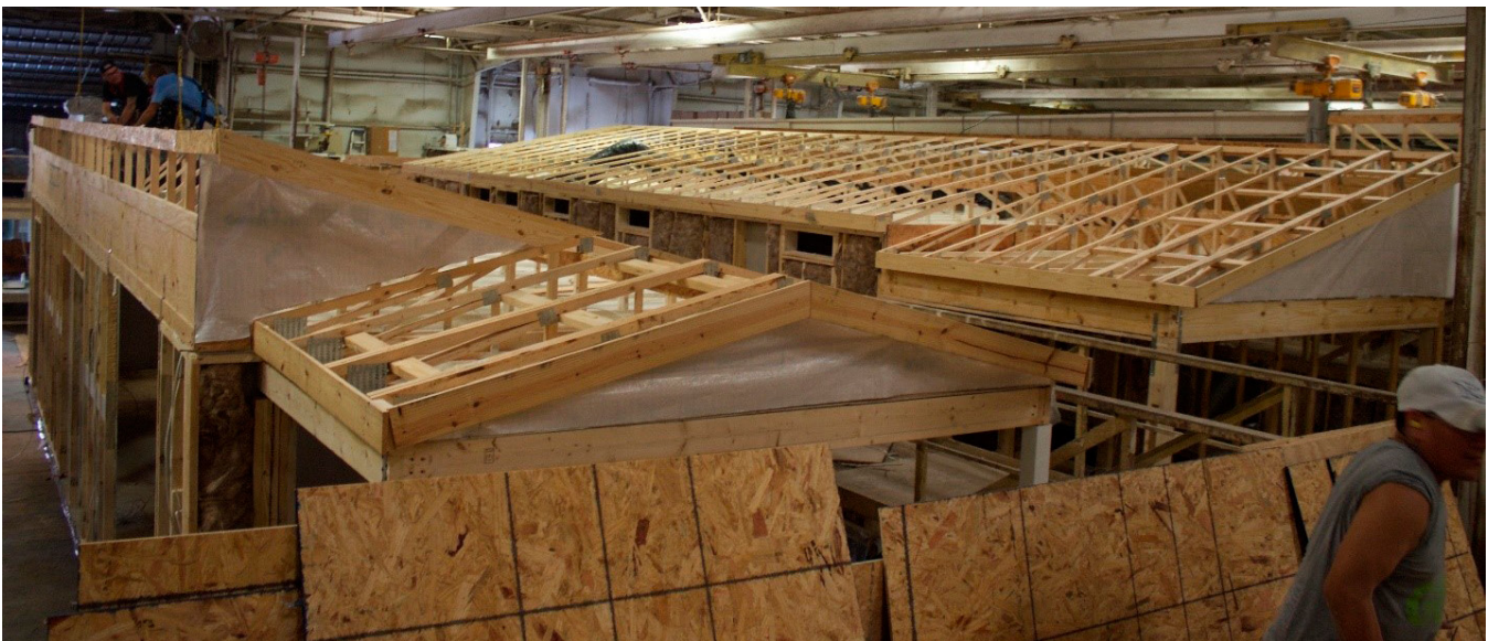
FIGURE 1.43, 1.44, 1.45, AND 1.46: THE ROOF IS SET ONTO THE WALLS AND SQUARED AND FASTENED PROPERLY.
