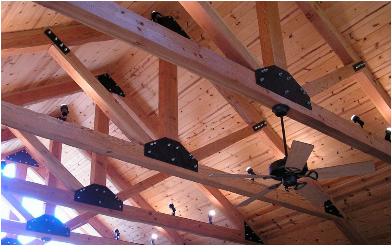
FIGURE 1.38: THE ROOF SUPPORT SYSTEM IN THIS HOME IS MADE UP OF TRUSSES THAT ARE ENGINEERED AND MANUFACTURED BY SPECIALIZED TRUSS MANUFACTURERS.
