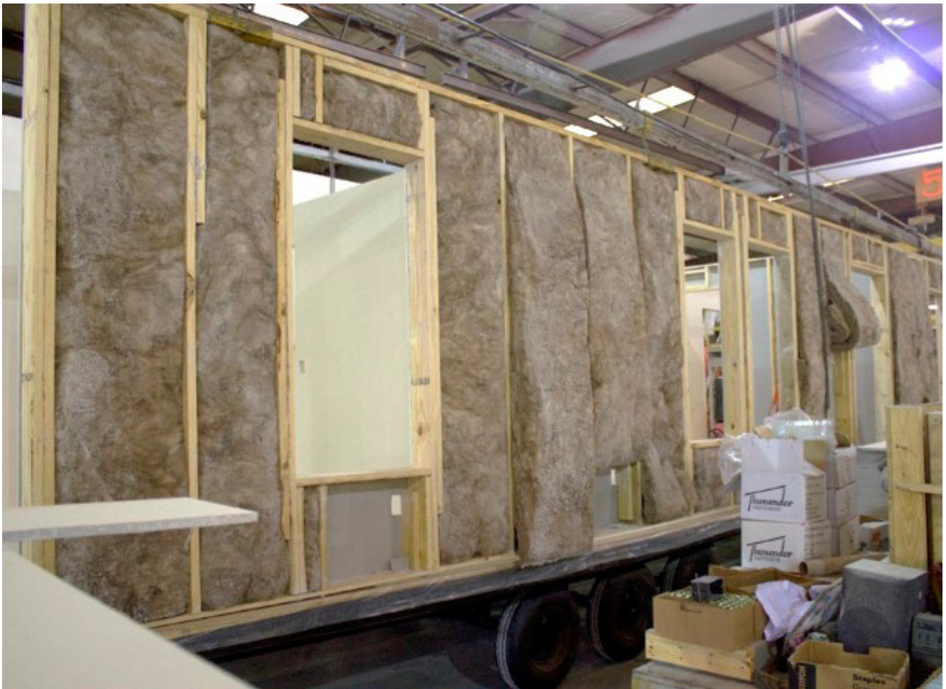
FIGURE 1.31, 1.32: THE SIDE WALL IS BUILT IN THE OFFLINE STATION AND THEN SET ON THE ONLINE PRODUCTION LINE.
