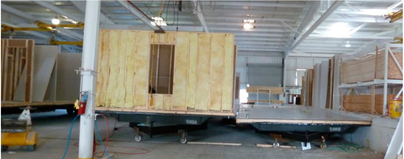
FIGURE 1.6: THE CHASSIS IS USED TO SUPPORT AND TRANSPORT THE HOME TO ITS FINAL DESTINATION.
