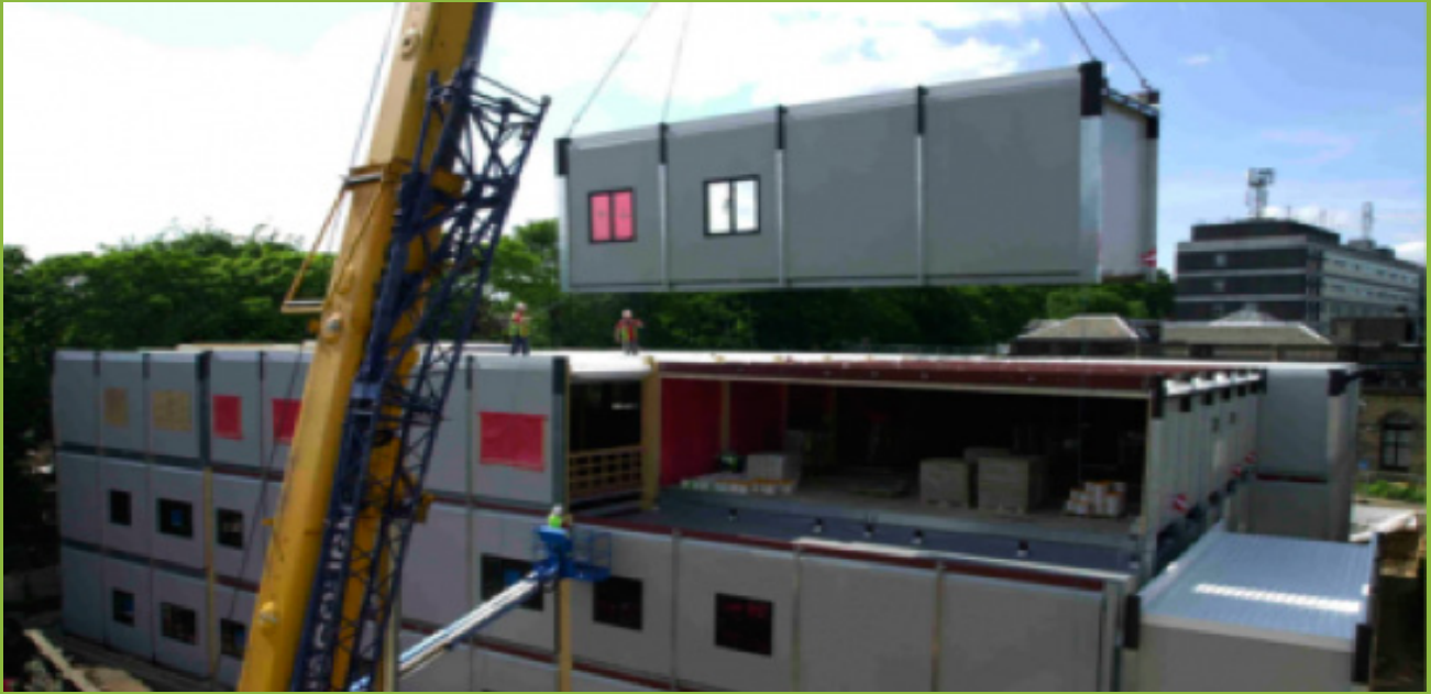
FIGURE 1.20: MODULAR HOSPITAL BUILDING INSTALLATION OF OPEN SIDED MODULES (IMAGE COURTESY OF YORKON)
