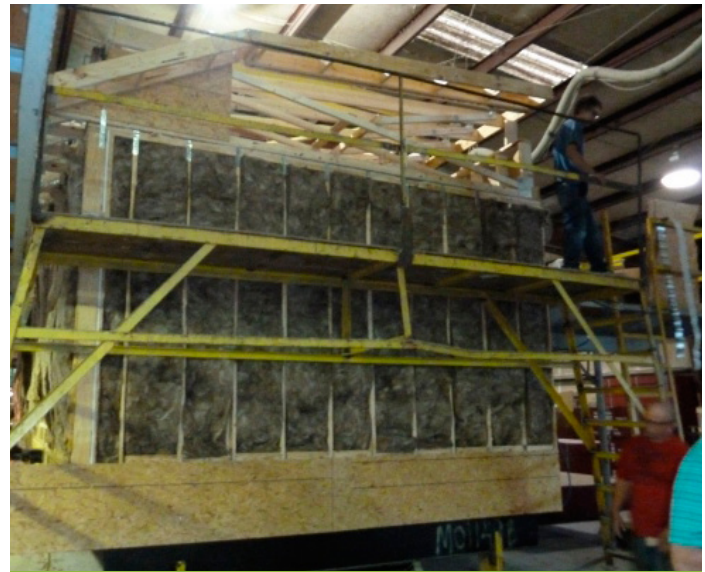
FIGURE 2.9: USE OF GANTRIES IN THE FACTORY
