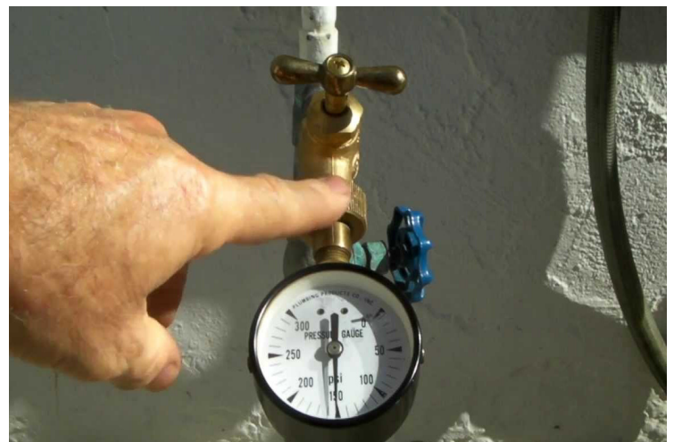
FIGURE 2.33 A PRESSURE GAUGE IS USED TO TEST WATER PRESSURE IN THE SYSTEM.
