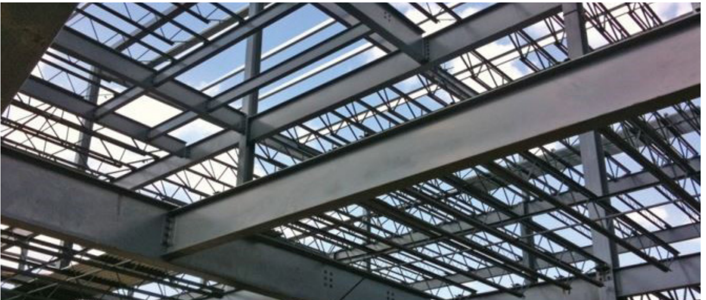
FIGURE 3.25 - A CONVENTIONAL METAL STRUCTURE IS READY TO BE COMPLETED WITH METAL SYSTEMS ENCOMPASSING ALL CONVENTIONAL STEEL PRODUCTS — RANGING FROM WIDE-FLANGE BEAMS AND BAR JOISTS TO PIPES AND TUBES. THIS PRODUCTION IS A GOOD EXAMPLE OF THE KIT-OF-PARTS APPROACH WHERE ALL PARTS ARE STANDARDIZED. (SOURCE: BUTLER MANUFACTURING)
