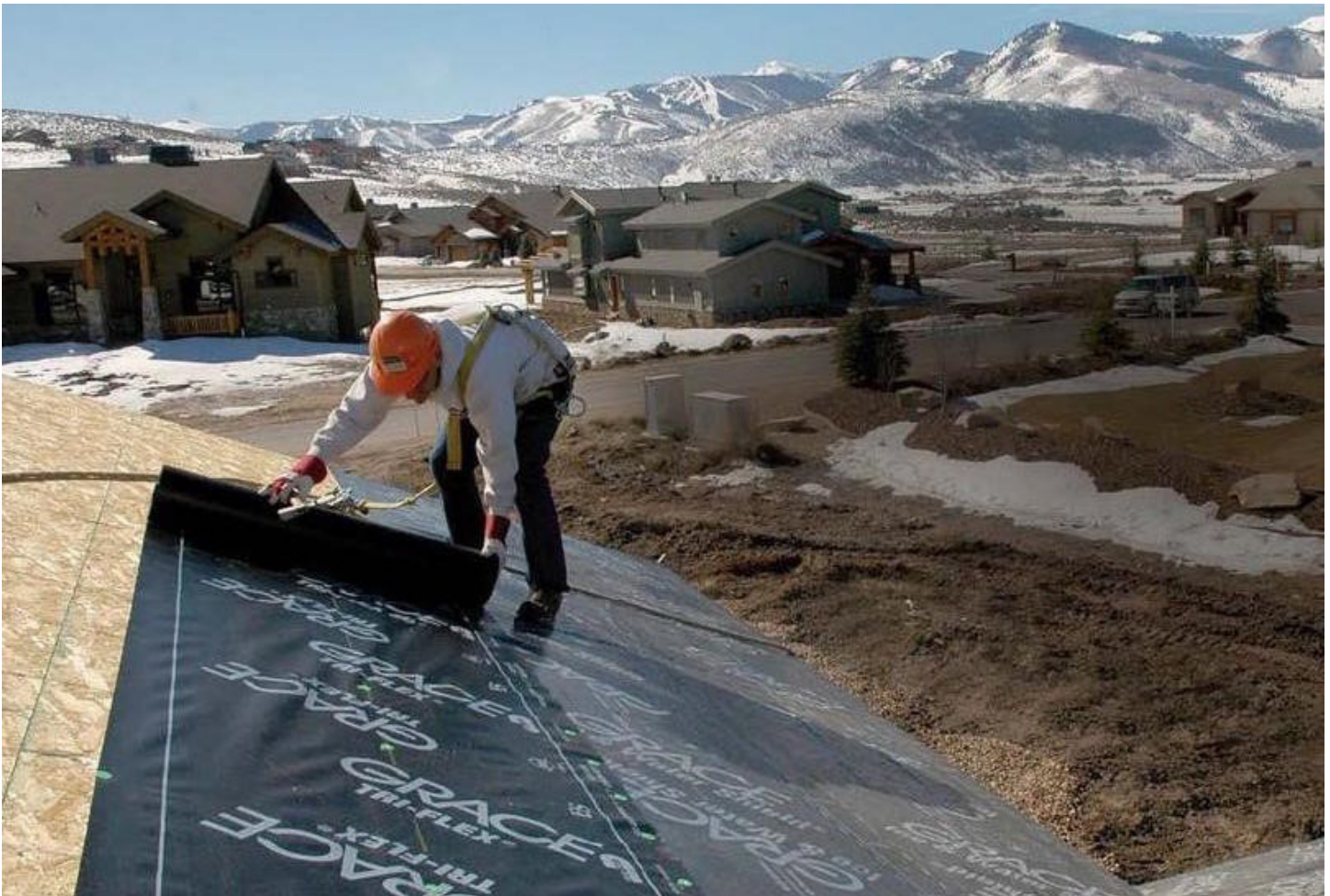
FIGURE 2.3 ASPHALT FELT ROLL INSTALLATION STARTS AT LOWER CORNER. THE FELT SHOULD HAVE AT LEAST 2" TOP LAP OVER THE LOWER COURSE AND 4" END LAP. NAILING IS REQUIRED EACH 16" OVER EACH LAPS AND CENTER OF EACH LAYER. (SOURCE: HOME DEPOT PRODUCT AUTHORITY)
