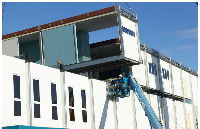
FIGURE 3.16 - TECHNICALLY ADVANCED MODULAR STEEL INSTALLATION: THE MODULES CAN BE STACKED VERTICALLY AND HORIZONTALLY ON ONE ANOTHER. THE FLOOR AREA CAN BE THEREFORE REDUCED OR INCREASED BASED ON THE REQUIRED PROGRAM. (SOURCE: WWW.DESIGNINGBUILDINGS.CO.UK)
