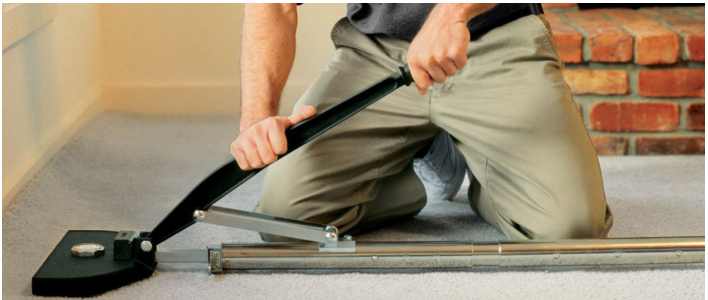
FIGURE 2.12 A POWER STRETCHER IS USED FOR CARPET INSTALLATION IN THE STRETCH-IN METHOD. (SOURCE: ARSLANIAN BROS.)
