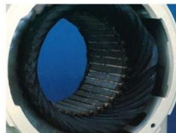
Overload damage to all windings Note: Under-voltage and over-voltage (exceeding NEMA standards) will result in the same type of insulation deterioration.
