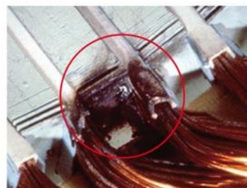
Winding grounded at edge of slot (caused by contamination, abrasion, vibration, or voltage surge)
