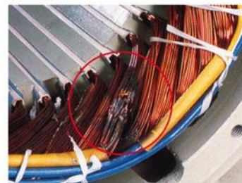
Voltage surge damage (caused by lightning, capacitor discharges, voltage kickbacks caused by de-energizing large inductive loads, or voltage disturbances caused by solid-state devices)
