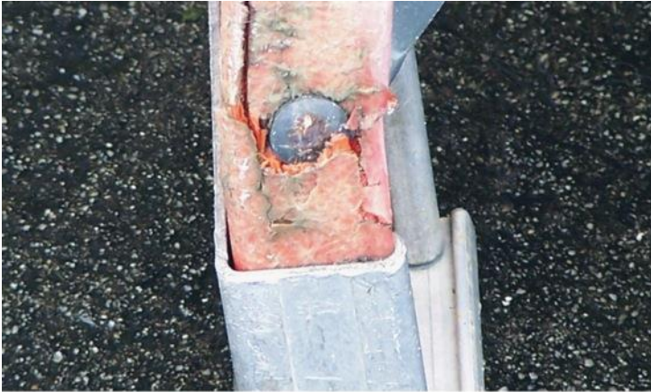
(A) CRUMBLING RAIL
