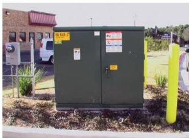
(A) PAD-MOUNTED COMMERCIAL TRANSFORMER
