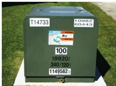
(A) PAD-MOUNTED TRANSFORMER
