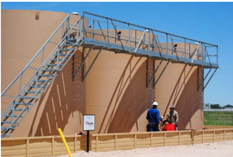
Photo 2: Contractors complete site work to NMJC's new Oil & Gas Training Ground in preparation for new trainings starting this summer.
