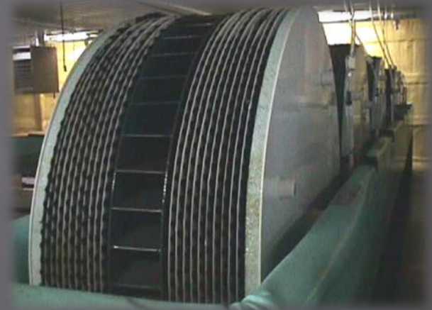
In-tank RBC airlift driven
