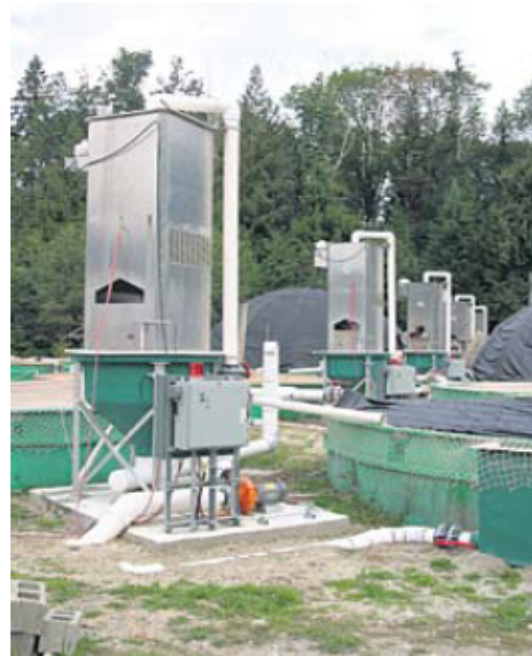
Phase 1. Partial re-use treatment systems showing tank connection, pump, and gas transfer tower.
