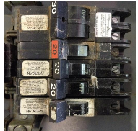
Circuit Breakers in a Breaker Panel
