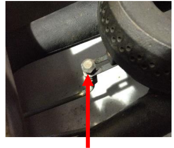
Pilot Light next to burner
