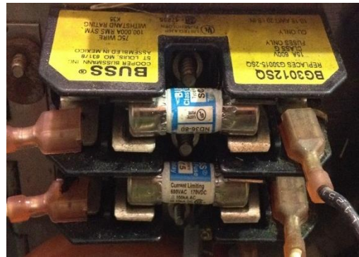
Fuses on a Conveyor Oven
