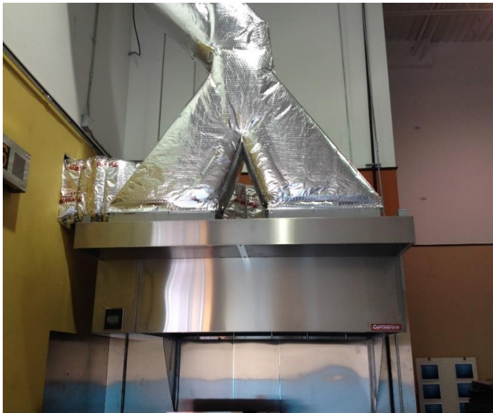
Commercial Ventilation System
