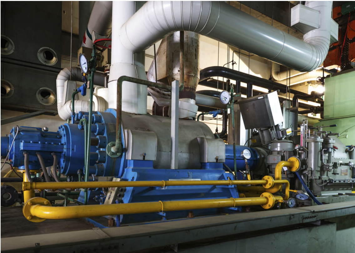
Figure 4-1: A boiler provides heating for a facility. (Source: hxdyl/iStock/Thinkstock)
