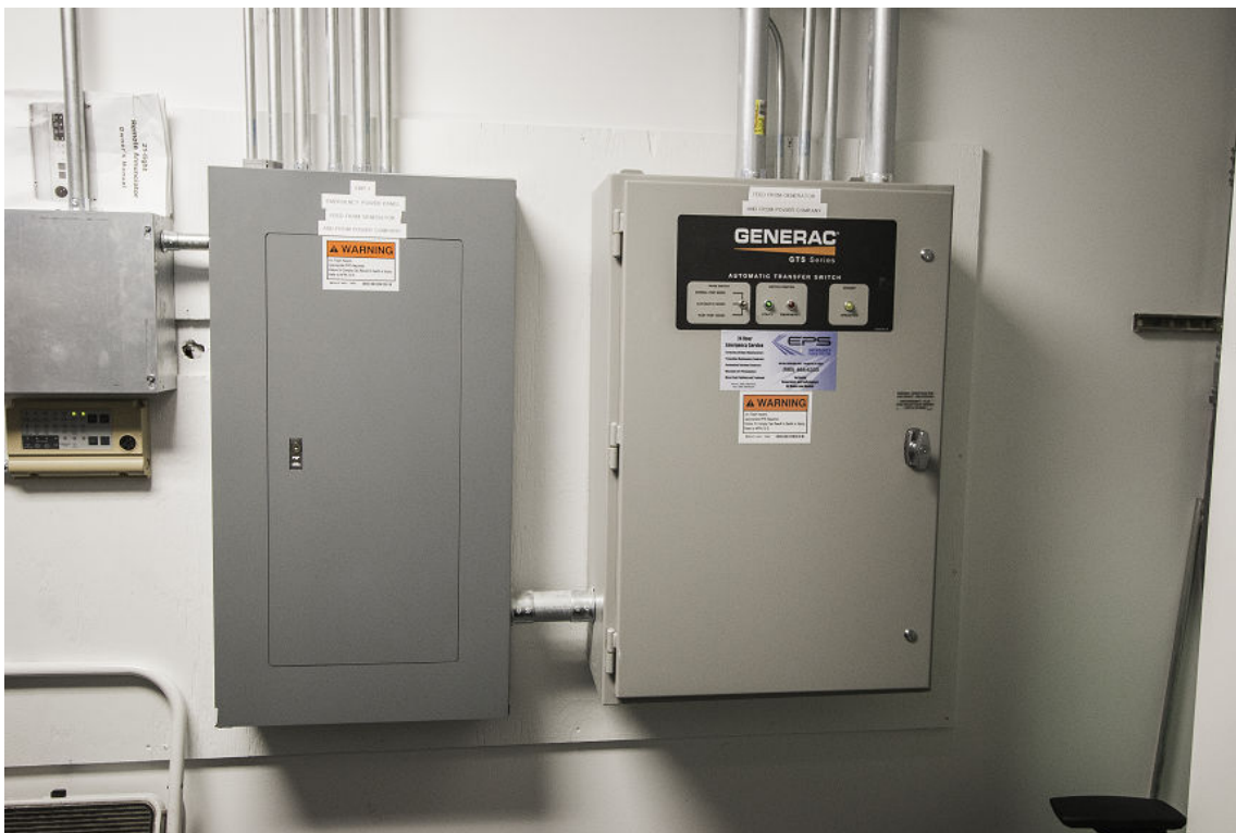
Figure 3–4: An automatic transfer switch connected to the main breaker box. (Source: Logical Operations for NCMCO)
