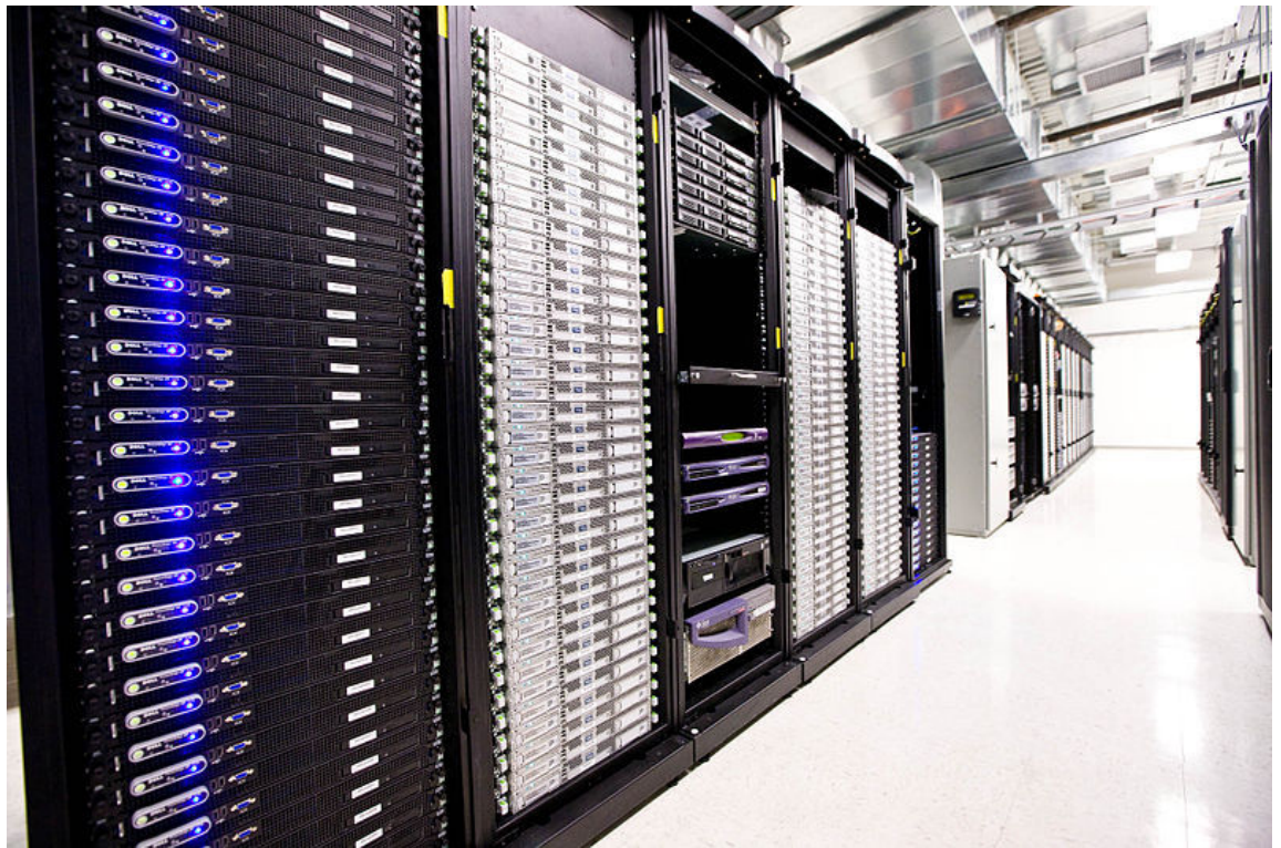
Figure 1–2: Server racks in a data center, which is often the heart of IT infrastructure for a facility. (Source: Global Access Point/Creative Commons (Public Domain)/ https://commons.wikimedia.org/wiki/File:Inside_Suite.jpg )
