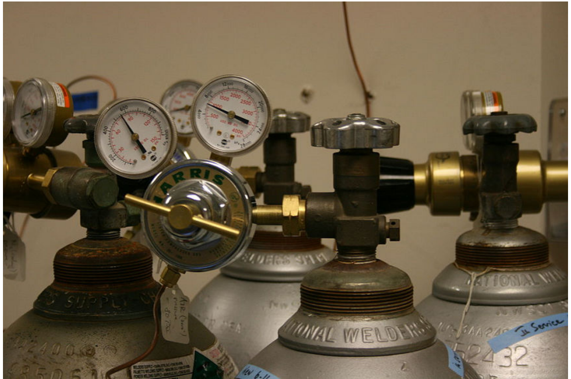
Figure 12–7: Pressure regulators and gauges installed on various compressed gas storage containers. (Source: Ildar Sagdejev/Creative Commons (CC BY-SA 3.0)/ https://commons.wikimedia.org/wiki/File:2008-07-02_Pressure_regulators.jpg )
