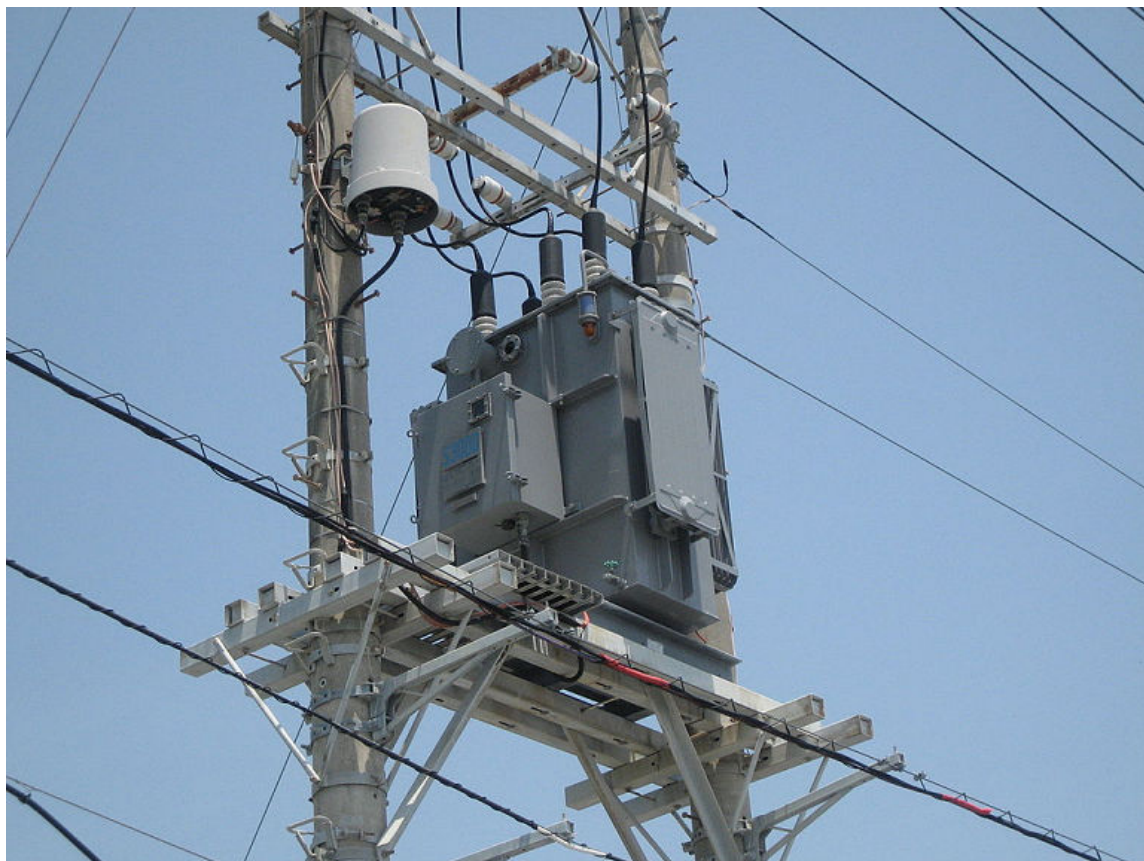
Figure 2–2: The equipment that is part of the utility supply, such as a step voltage regulator, operates using high voltage. (Source: Ebiebi2/Creative Commons (Public Domain)/ https://commons.wikimedia.org/wiki/File:Step_Voltage_Regulator_1.JPG )
