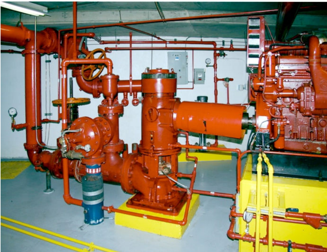
Figure 6-7: A fire pump system helps move water quickly and efficiently to the location of the fire. (Source: Toddastephens/Creative Commons (CC BY-SA 3.0)/ https://commons.wikimedia.org/wiki/File:Vertturbdsfirepump.jpg )
