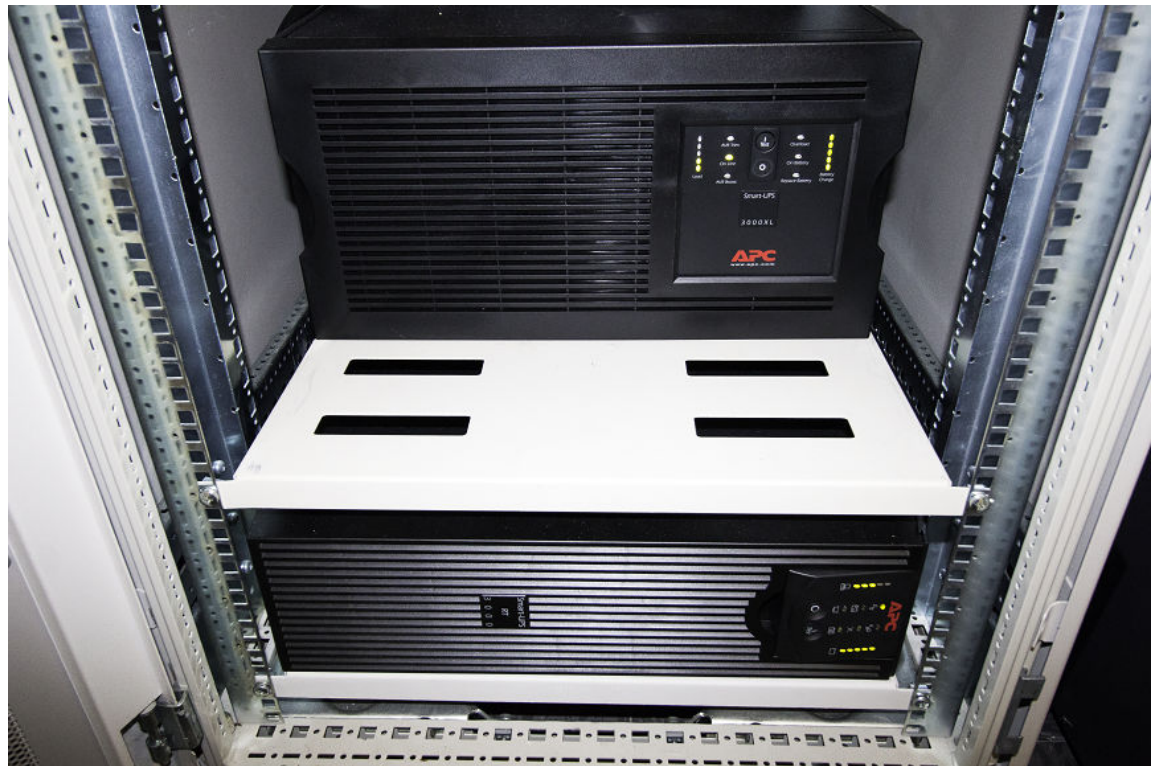
Figure 2–13: A UPS on server racks in a small-scale data center. (Source: Logical Operations for NCMCO)
