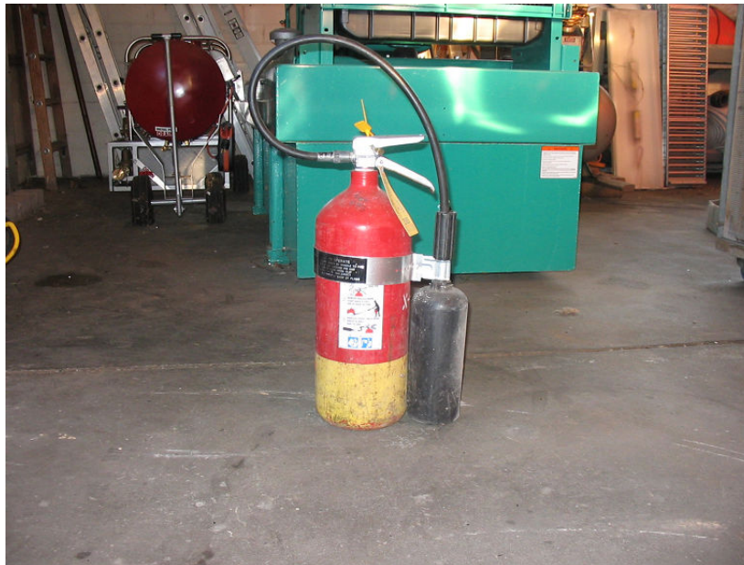
Figure 6–8: A CO 2 fire extinguisher. (Source: Rt66lt/Creative Commons (CC BY-SA 3.0)/ https://commons.wikimedia.org/wiki/File:CO_extinguisher_2.PNG )
