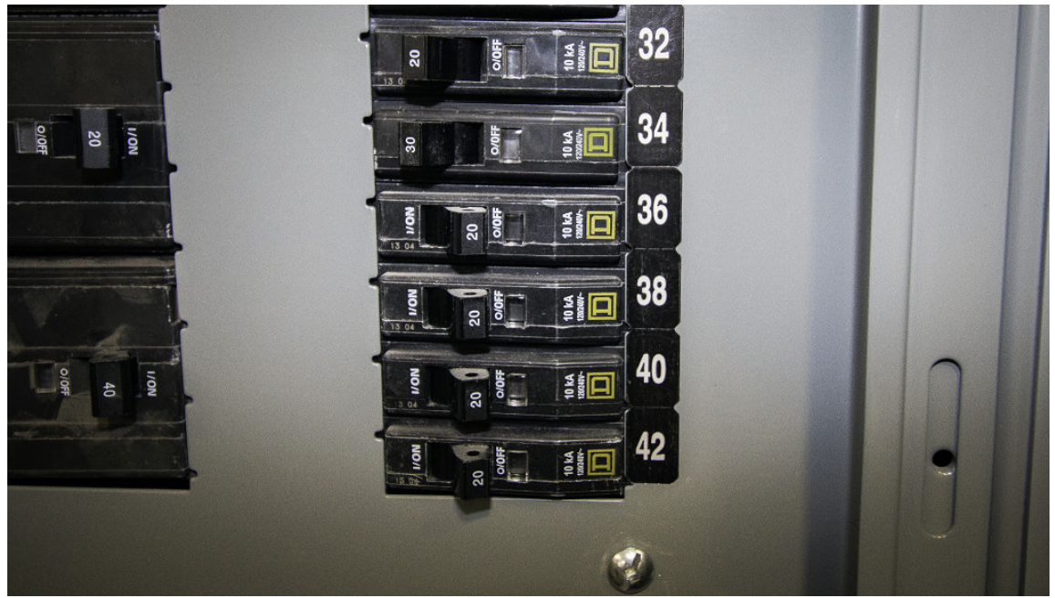
Figure 3–10: In over-current protection, a breaker automatically switches to the off position when the power exceeds the level it can support. (Source: Logical Operations for NCMCO)
