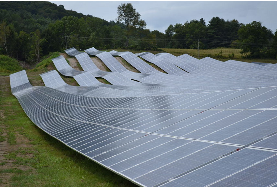
Figure 2-17: Long rows of solar panels on a solar farm in Sharon, Vermont. (Source: SayCheeeeeese/Creative Commons (Public Domain)/ https://commons.wikimedia.org/wiki/File:SunGen_Sharon_Solar_7.jpg )
