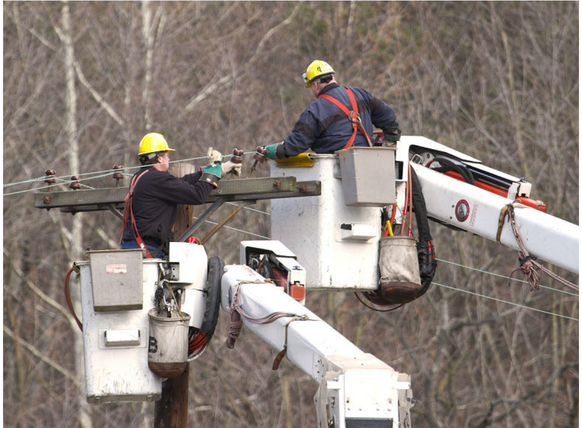
Figure 13–7: Two linemen follow the double custody switching protocol while performing maintenance on a power line. (Source: rpernell/iStock/Thinkstock)
