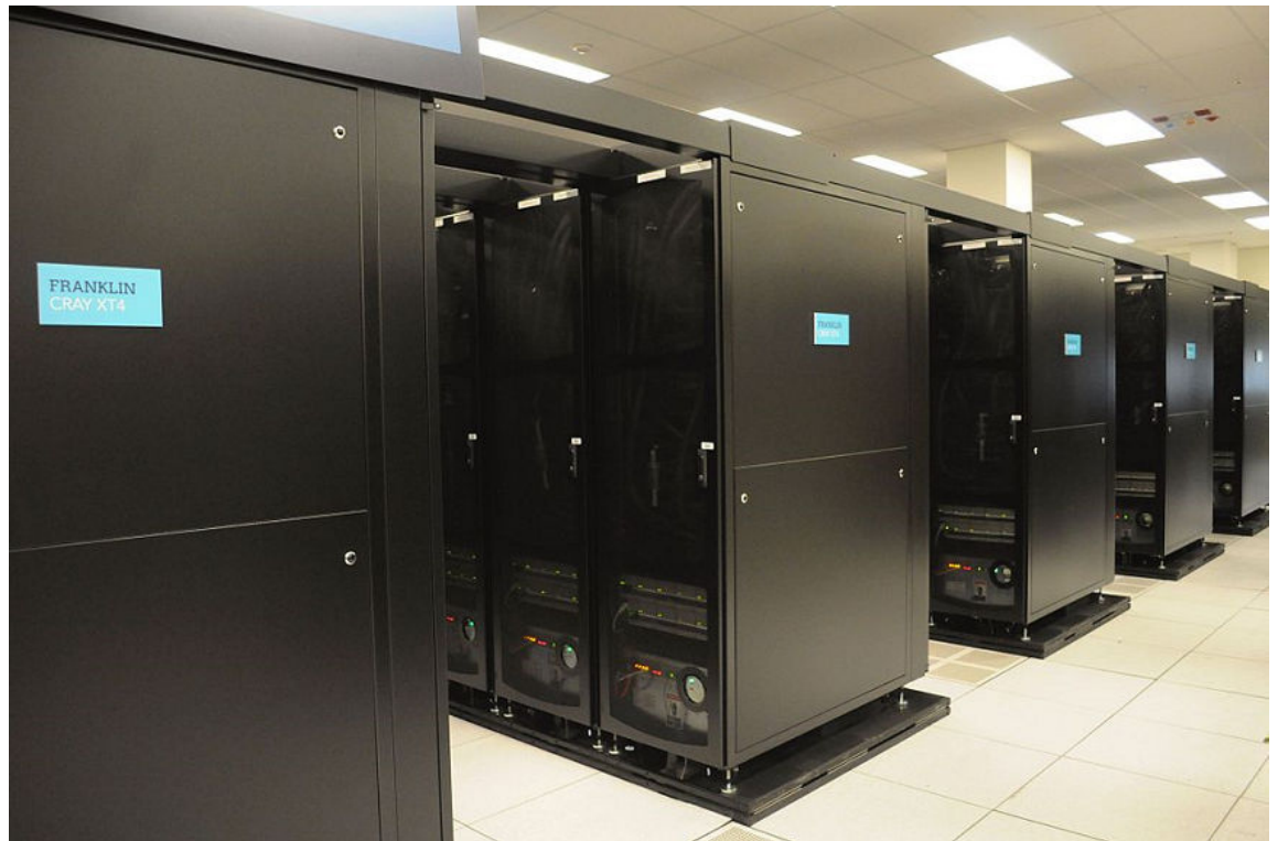
Figure 9–1: Server racks, which can be numerous, need to be well-placed in the data center. (Source: Derrick Coetzee/Creative Commons (Public Domain)/ https://commons.wikimedia.org/wiki/File:Rows_of_Franklin_Cray_XT4_racks.jpg )
