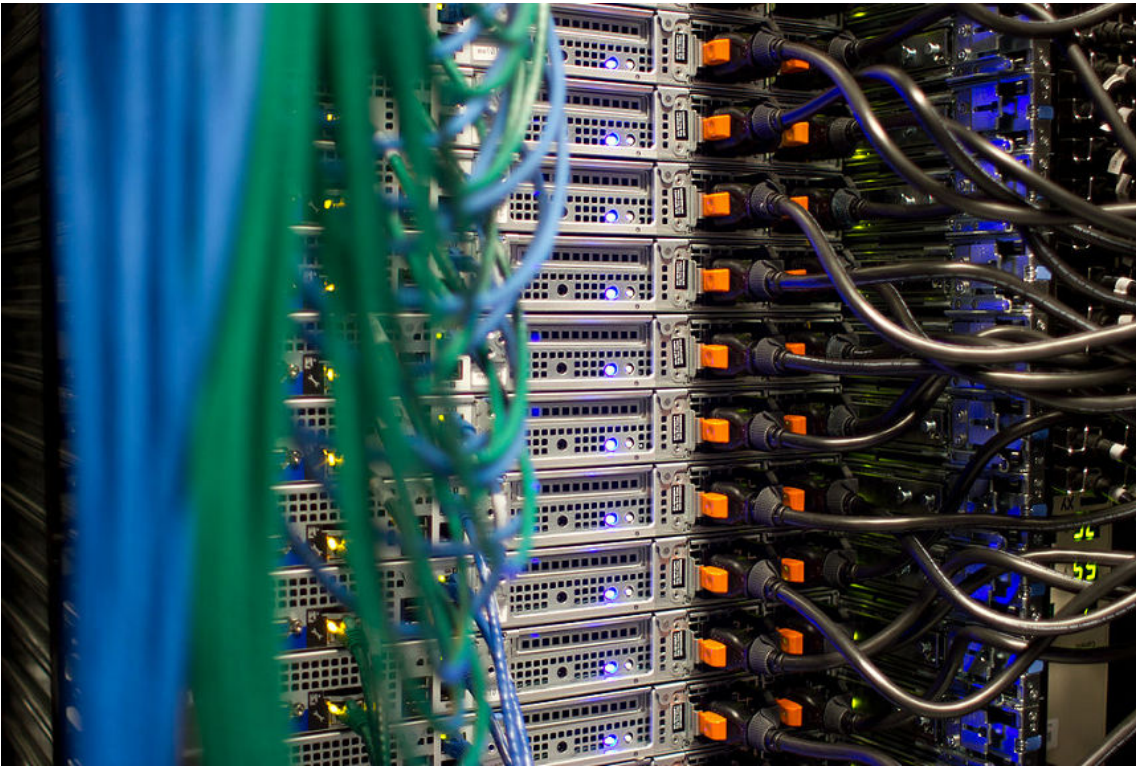
Figure 3-3: Rack-mounted servers in a data center utilize dual-cord supplies to provide power redundancy. (Source: Victorgrigas/Creative Commons (CC BY-SA 3.0)/ https://commons.wikimedia.org/wiki/File:Wikimedia_Foundation_Servers-8055_24.jpg )
