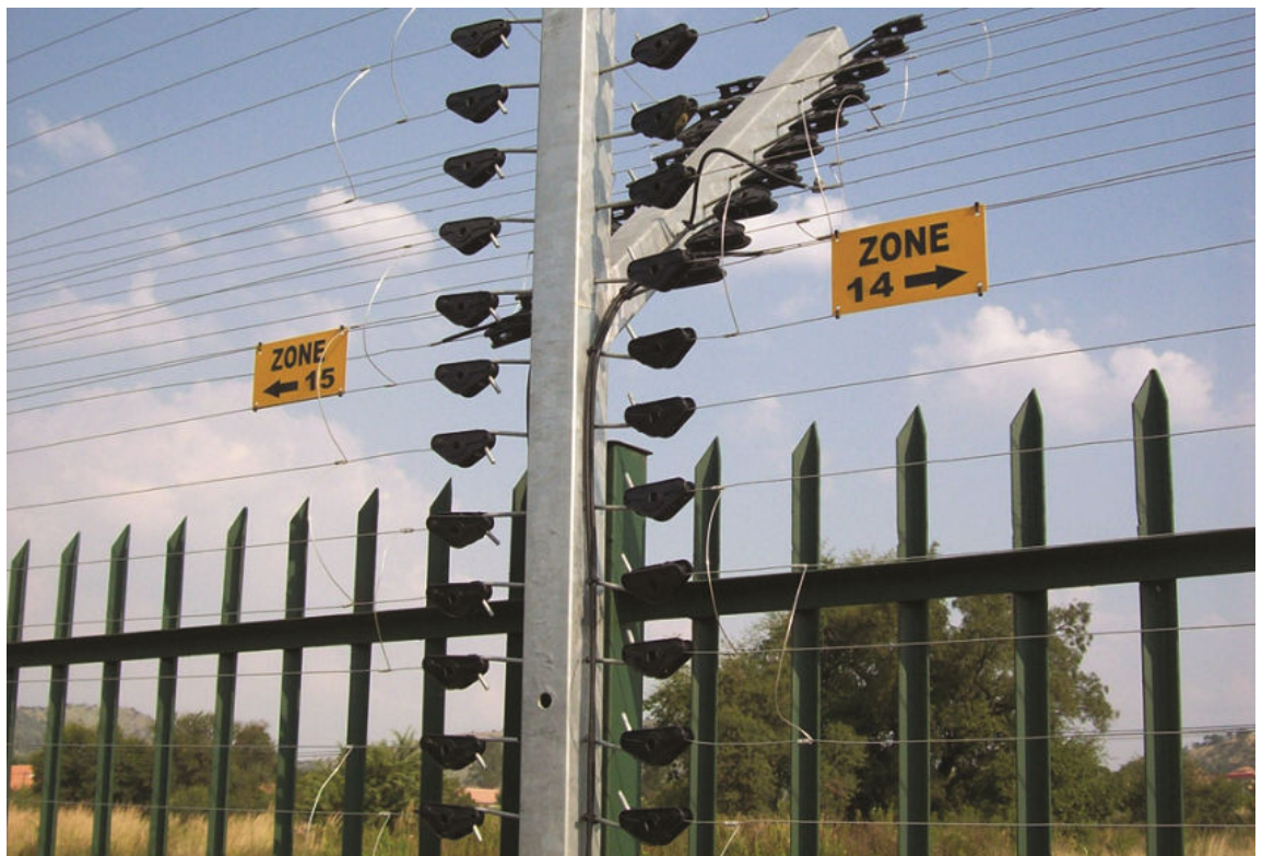
Figure 8-3: A multi-zone electrical fence installed on top of other fencing serving as a physical barrier to entry. (Source: PaktonDale/Creative Commons (CC BY-SA 4.0)/ https://commons.wikimedia.org/wiki/File:Security_Electric_Fence.JPG )
