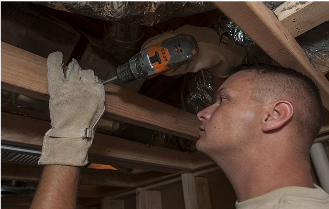
Figure 13–10: An HVAC technician installs HVAC vents using ASHRAE's standards and guidelines. (Source: United States National Guard/Creative Commons (Public Domain)/ https://commons.wikimedia.org/wiki/
