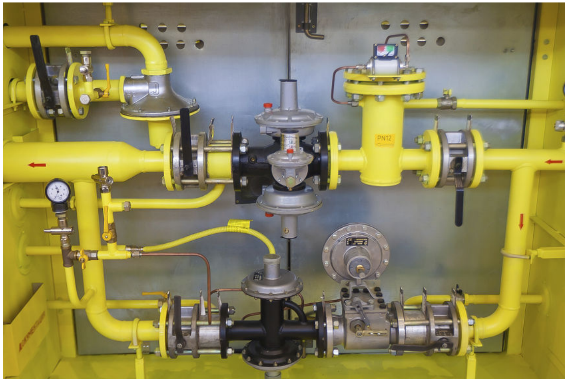
Figure 5–7: Natural gas pipes and valves in a building. (Source: tdhster/iStock/Thinkstock)
