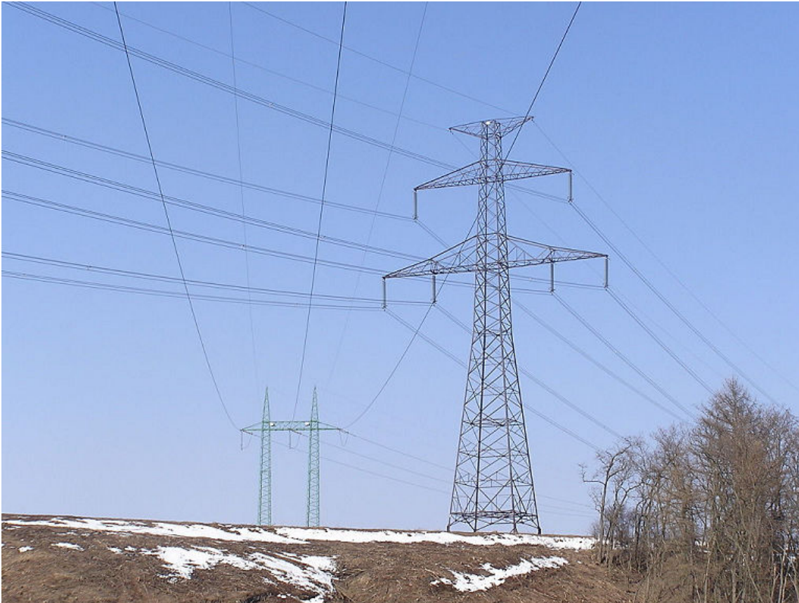
Figure 2-1: Power lines provide the type of electricity we are most familiar with: the kind that provides power to our homes and businesses. (Source: Jan Dudik/Creative Commons (Public Domain)/ https://commons.wikimedia.org/wiki/File:Lec06m76.JPG )
