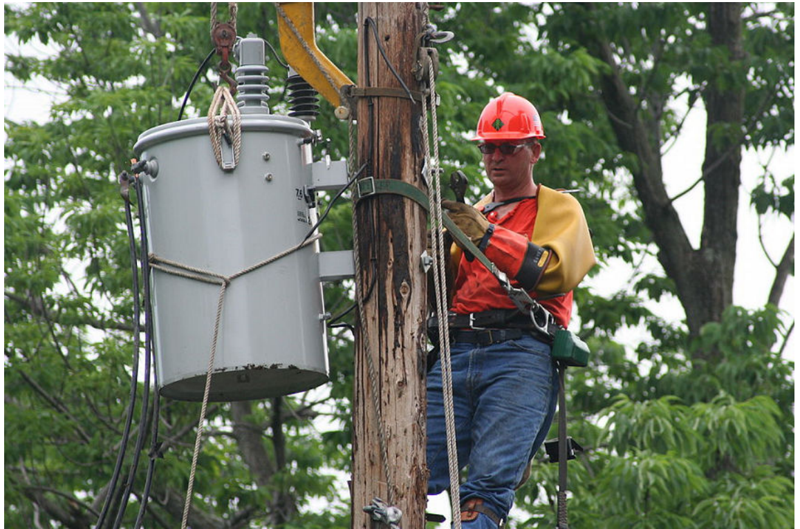
Figure 2–6: A utility lineman replaces the transformer on a utility pole, which decreases the high voltage coming along the power lines to a lower voltage that can be used in a home or business. (Source: Dave Pape/Creative Commons (Public Domain)/ https://commons.wikimedia.org/wiki/File:Lineman_changing_transformer.jpg )
