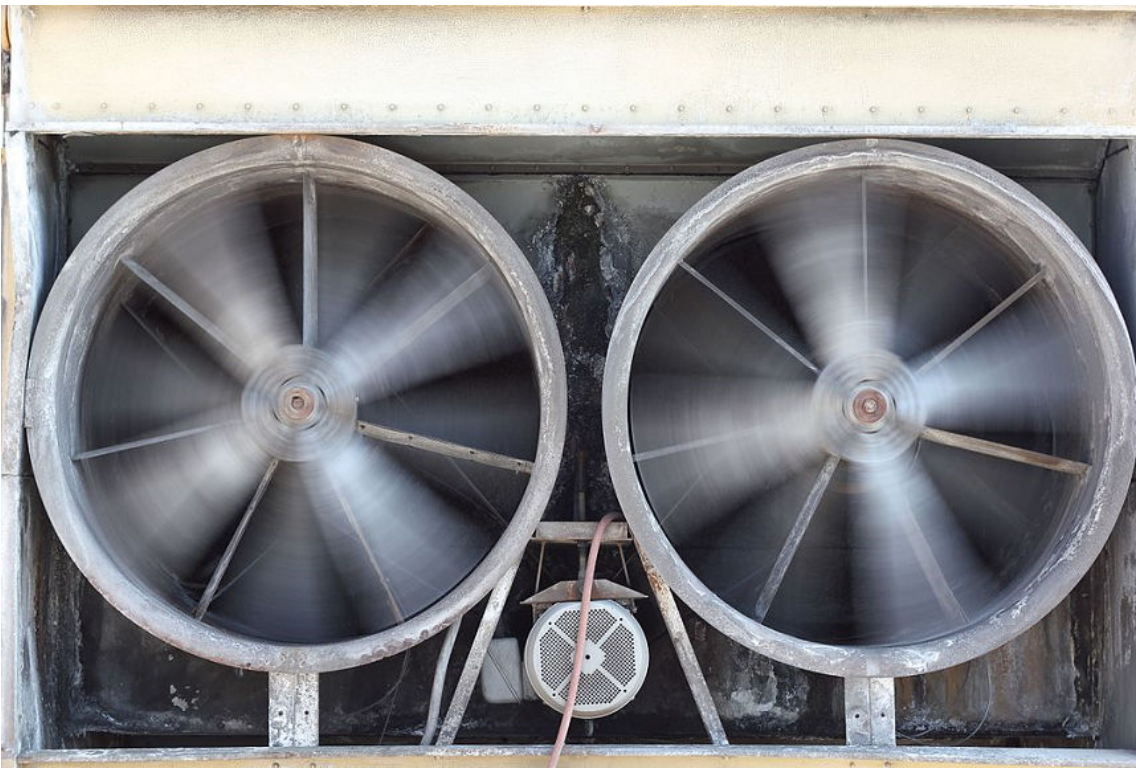
Figure 4-2: These large double-exhaust fans provide ventilation for an office building. (Source: PictorialEvidence/Creative Commons (CC BY-SA 3.0)/ https://commons.wikimedia.org/wiki/File:HVAC_Ventilation_Exhaust.jpg )
