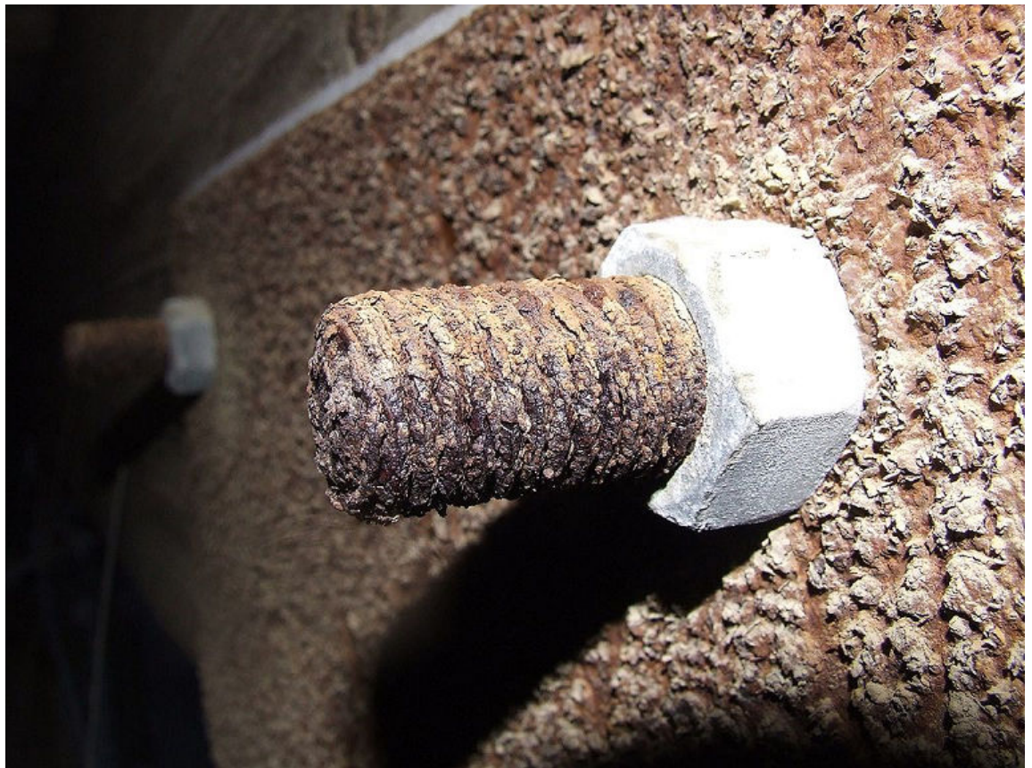
Figure 12–3: Corrosion, in the form of rust, on a metal bolt. (Source: Thester11/Creative Commons (CC BY-SA 3.0)/ https://commons.wikimedia.org/wiki/File:Rust_Bolt.JPG )
