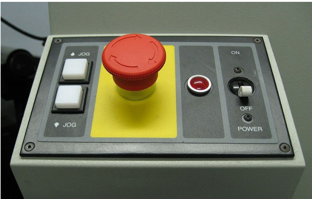
Figure 6–12: An EPO kill switch for a piece of machinery equipment in a laboratory. (Source: Cjp24/Creative Commons (CC BY-SA 3.0)/ https://commons.wikimedia.org/wiki/File:Emergency_stop_button.jpg )
