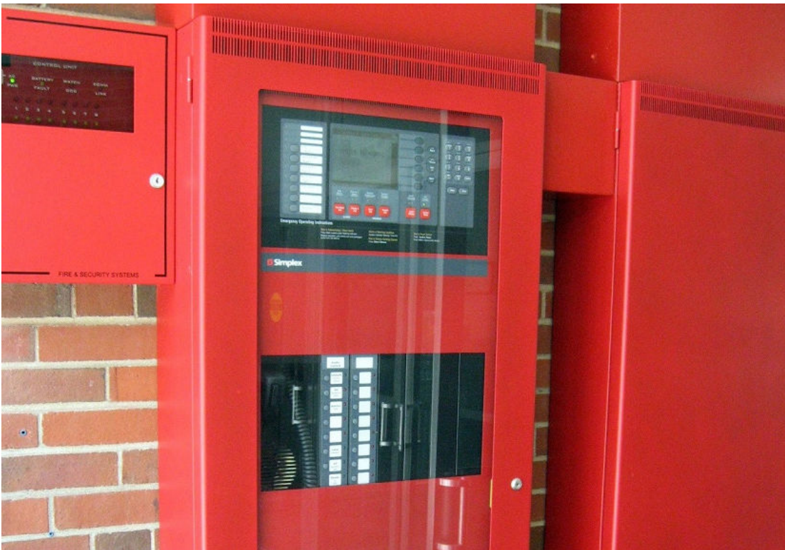
Figure 6-5: A fire alarm control panel. (Source: Wile e2005/Creative Commons (CC BY 3.0)/ https://commons.wikimedia.org/wiki/File:Simplex4100Upnel.JPG )
