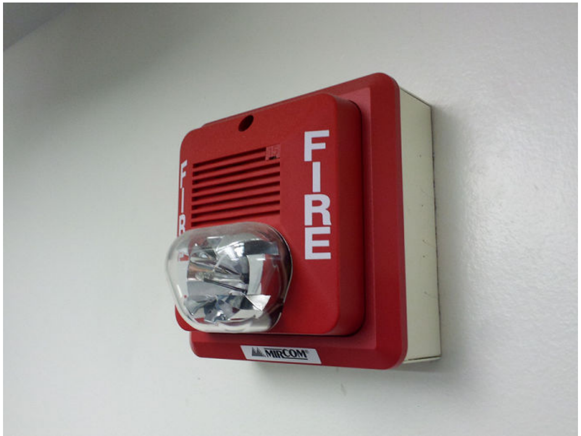
Figure 6-4: The speaker and strobe light of a fire alarm system. (Source: Ben Schumin/Creative Commons (CC BY-SA 2.0)/ https://commons.wikimedia.org/wiki/File:Mircom_Fire_Alarm_HornStrobe.jpg )
