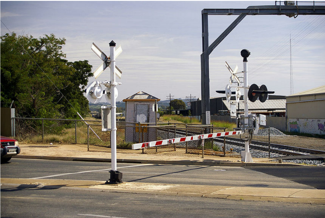
Figure 8–4: Boom barriers prevent vehicles from entering a restricted area without permission. (Source: Bidgee/Creative Commons (CC BY-SA 3.0)/ https://en.wikipedia.org/wiki/File:Bourke-Docker_Street_level_crossing_boom_gate.jpg )
