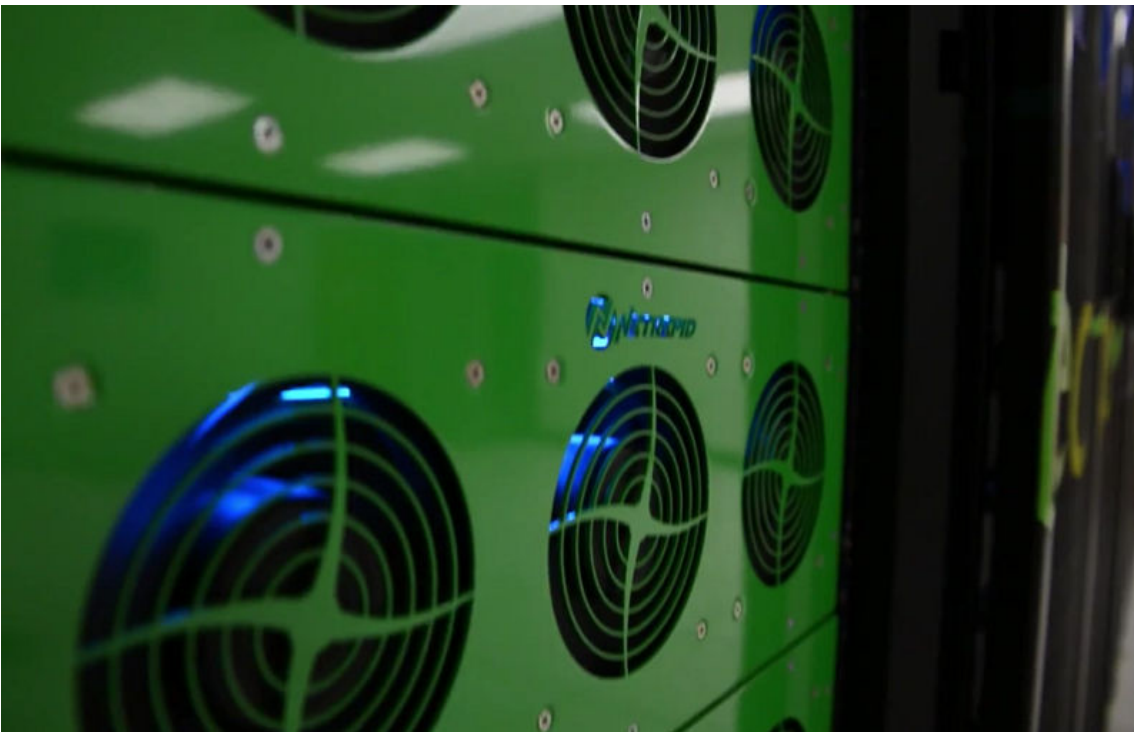
Figure 9–3: The fans on a server rack are used to moderate the temperatures of the servers on the rack. (Source: Annagen, LLC dba Netrepid/Creative Commons (CC BY-SA 3.0)/ https://commons.wikimedia.org/wiki/File:Colocation_Cooling_Rack.png )
