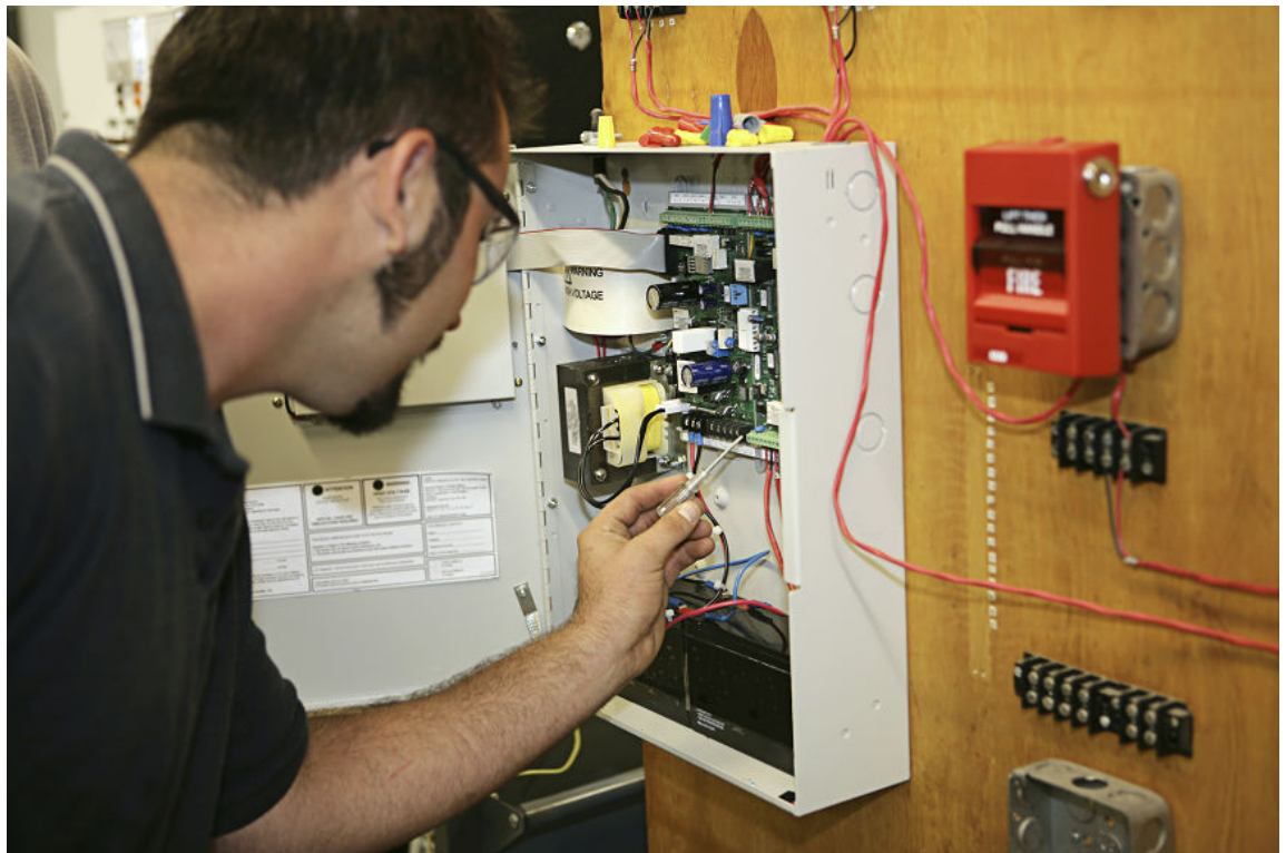
Figure 6–14: A certified technician performs maintenance tasks on a fire alarm control panel for a facility. (Source: Lisa F. Young/iStock/Thinkstock)
