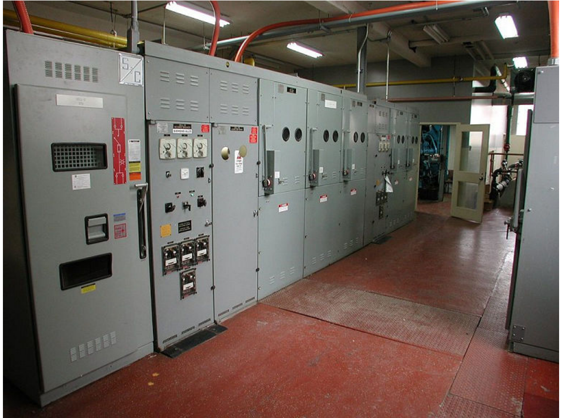
Figure 2–12: A paralleling switchgear in an MCO facility. (Source: P199/Creative Commons (Public Domain)/ https://commons.wikimedia.org/wiki/File:Electrical_switchgear.JPG )
