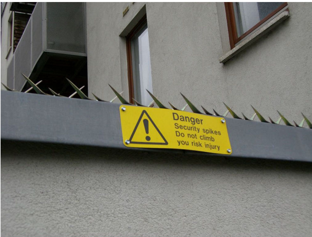
Figure 8-1: Both the sign and the spikes on this barrier wall indicate that unauthorized persons should not attempt to enter the secured space. (Source: Edward/Creative Commons (Public Domain)/ https://commons.wikimedia.org/wiki/File:Security_spikes_1.jpg )
