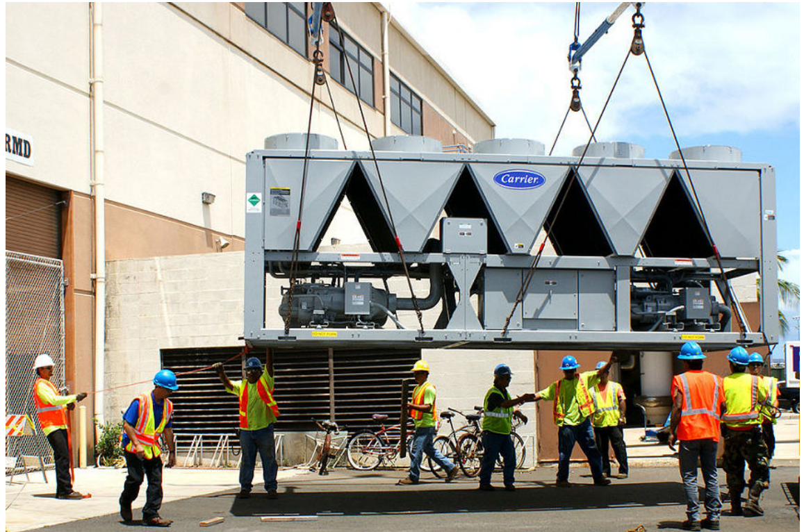
Figure 4-8: Workers guide a new air-cooled chiller into place for installation at a military base in Hawaii. (Source: United States Navy/Creative Commons (Public Domain)/ https://commons.wikimedia.org/wiki/File:US_Navy_100510-N-76290-003_New_air_conditioning_in_Hawaii.jpg )
