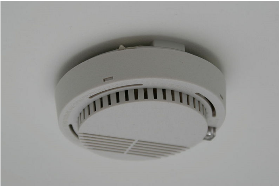
Figure 6–2: A typical smoke detector, installed on the ceiling. (Source: Tumi-1983/Creative Commons/CC BY-SA 3.0)/ https://commons.wikimedia.org/wiki/File:Smoke_detector.JPG
