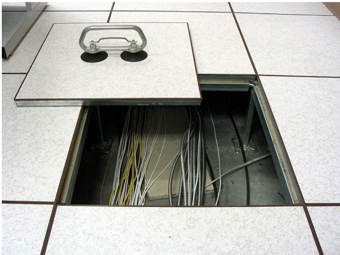
Figure 9–2: A floor tile is lifted out of the raised access flooring system to access the components below. (Source: Jonathan Lamb/Creative Commons (Public Domain)/ https://commons.wikimedia.org/wiki/File:Tile-lifter-in-use-raised-floor.jpg )
