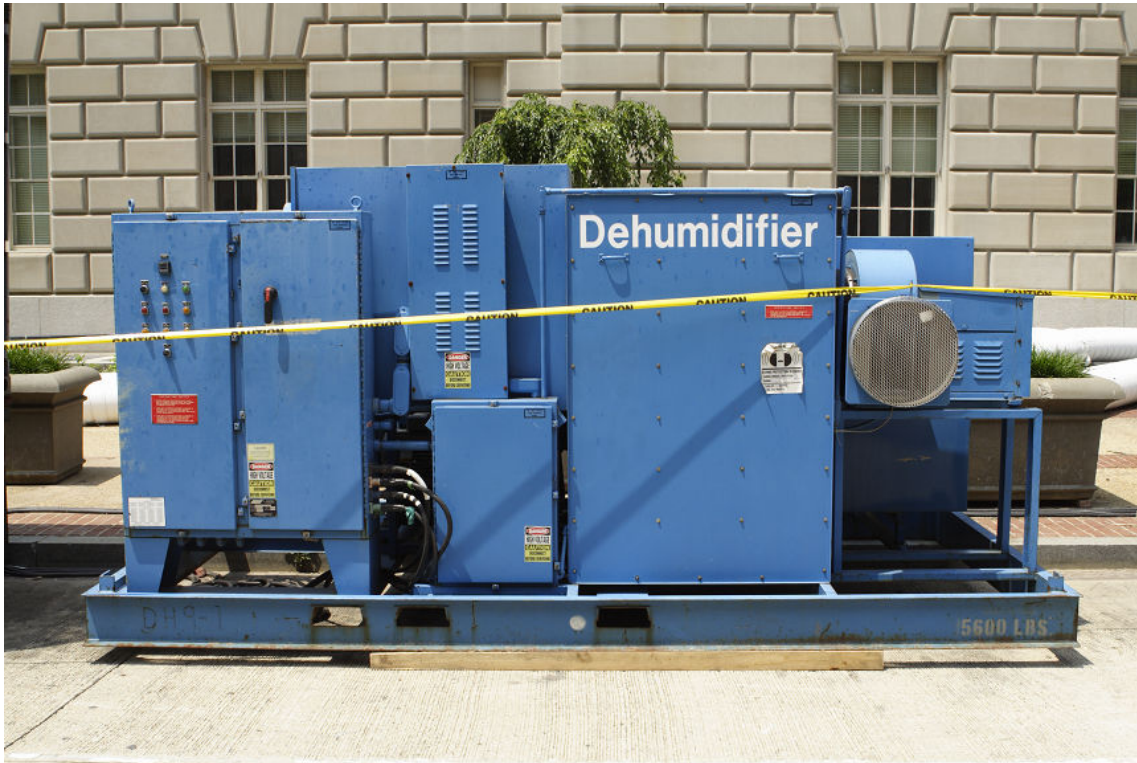
Figure 5-6: A large, industrial strength dehumidifier helps moderate the humidity levels for a building. (Source: jim pruit/iStock/Thinkstock)
