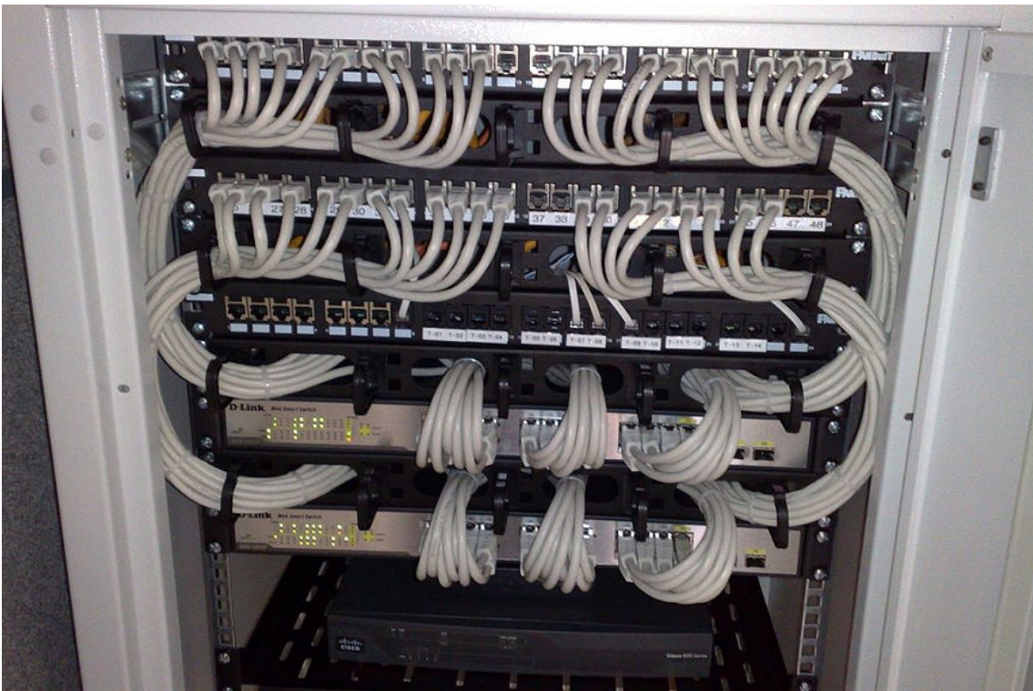
Figure 10-6: A series of rack-mounted switches (on the bottom) connected to patch panels (on the top) provide clean, organized cable management. (Source: Dsimic/Creative Commons (CC BY-SA 4.0)/ https://commons.wikimedia.org/wiki/File:19-inch_rackmount_Ethernet_switches_and_patch_panels.jpg )
