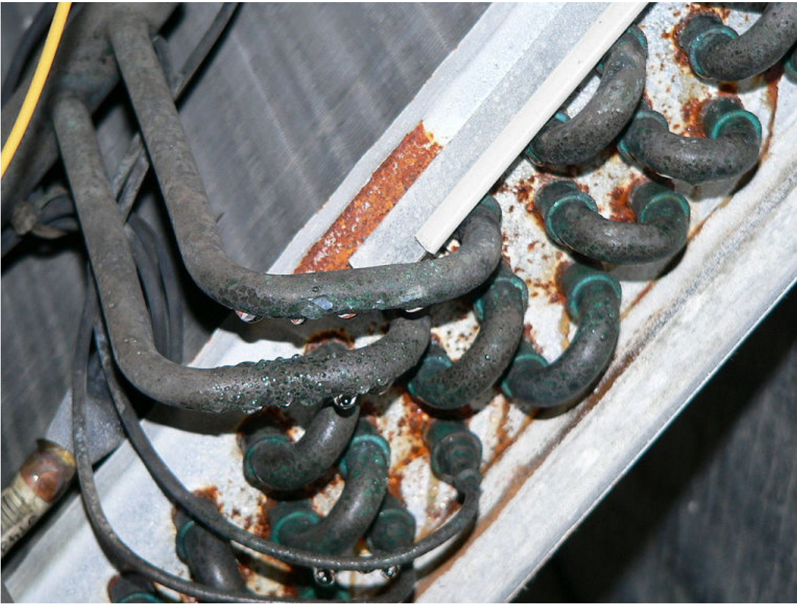
Figure 4-18: Corrosion can occur on evaporator coils if not properly maintained. (Source: Chinesedrywall/Creative Commons (CC BY-SA 3.0)/ https://commons.wikimedia.org/wiki/File:Effects_of_Chinese_Drywall.jpg )
