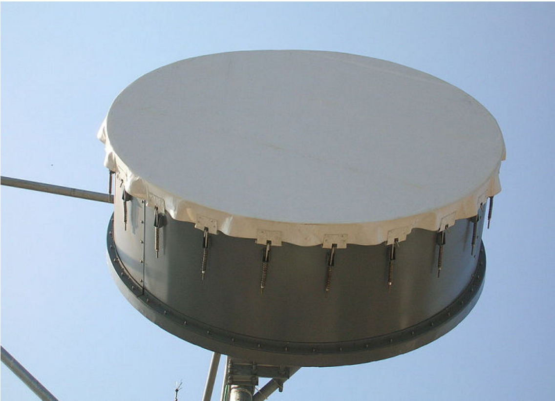
Figure 11-3: A microwave communications antenna. (Source: Faisal Akram/Creative Commons (CC BY-SA 2.0)/ https://commons.wikimedia.org/wiki/File: Microwave_Antenna_(2679399250).jpg )
