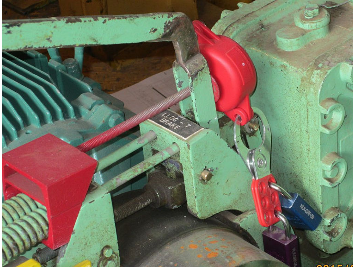
Figure 7-4: A lockout scissor clamp and two padlocks—one to secure the device, the other to prove it has been checked and verified—are applied to a hoist brake to prevent unexpected movement. (Source: Wtshymanski/Creative Commons (CC BY-SA 4.0)/ https://commons.wikimedia.org/wiki/File:Lockout_on_hoist_brake.JPG )
