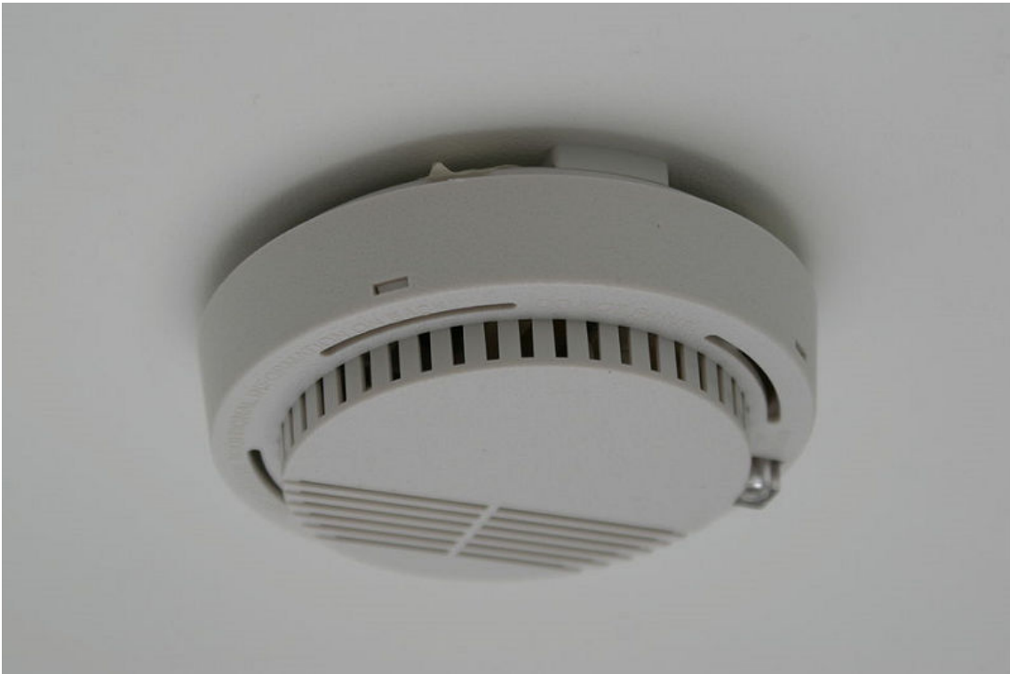
Figure 6–2: A typical smoke detector, installed on the ceiling. (Source: Tumi-1983/Creative Commons/CC BY-SA 3.0)/ https://commons.wikimedia.org/wiki/File:Smoke_detector.JPG
