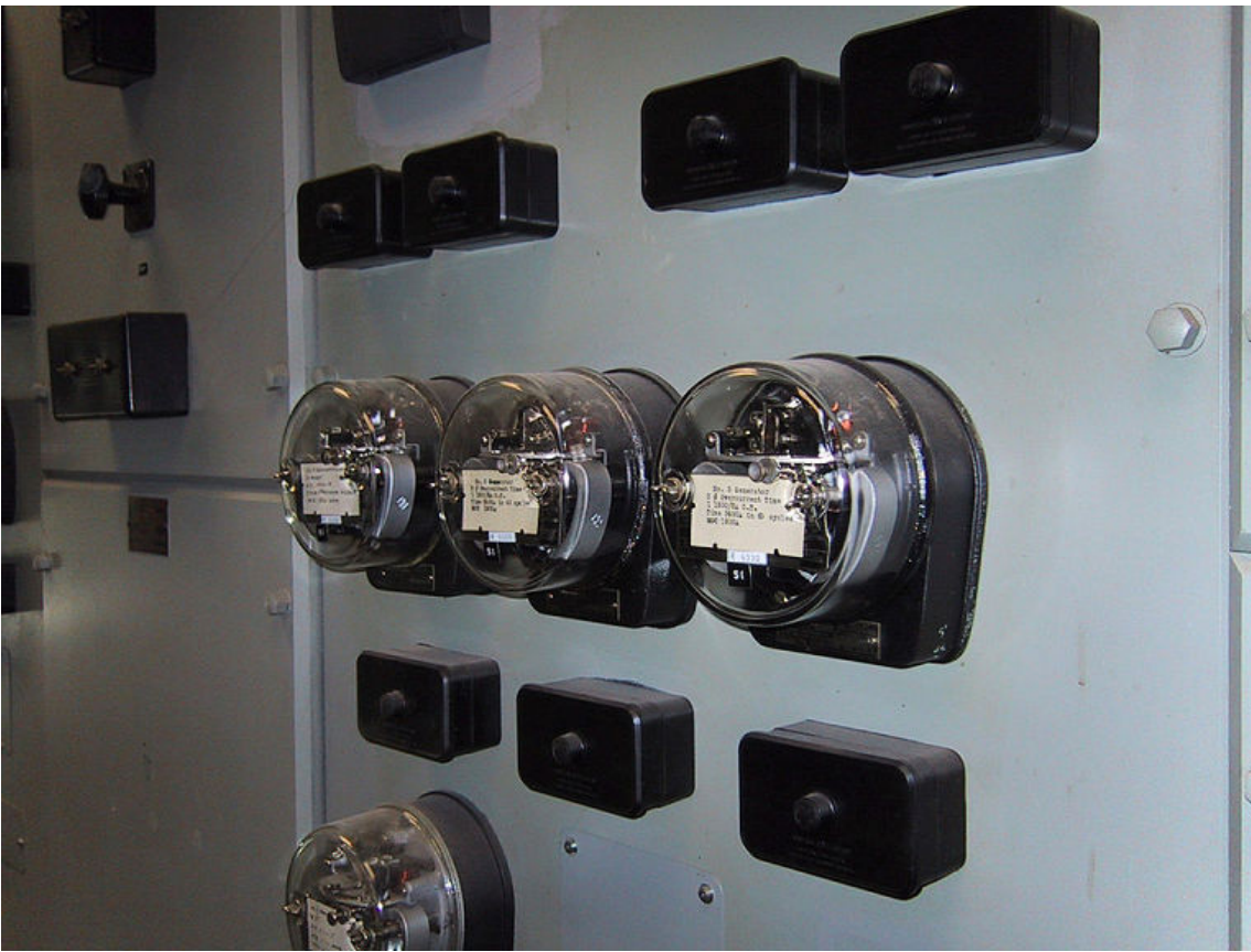
Figure 3-11: Protective relays used to provide over-current protection at a power generating station. (Source: Wtshymanski/Creative Commons (CC BY-SA 3.0)/ https://commons.wikimedia.org/wiki/File:Protective_Relays_Hydroelectric_Station.JPG )
