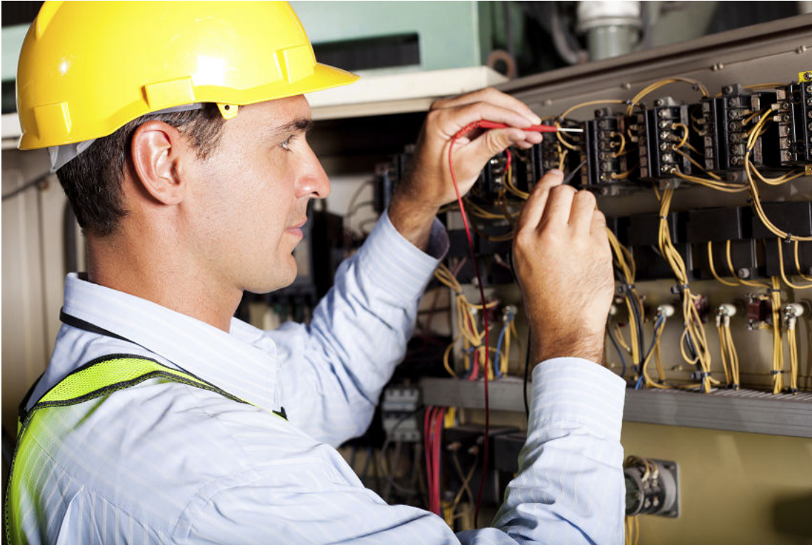
Figure 1-16: An electrician, as part of the operations team for a facility, works on an electric panel. (Source: michaeljung/iStock/Thinkstock)
