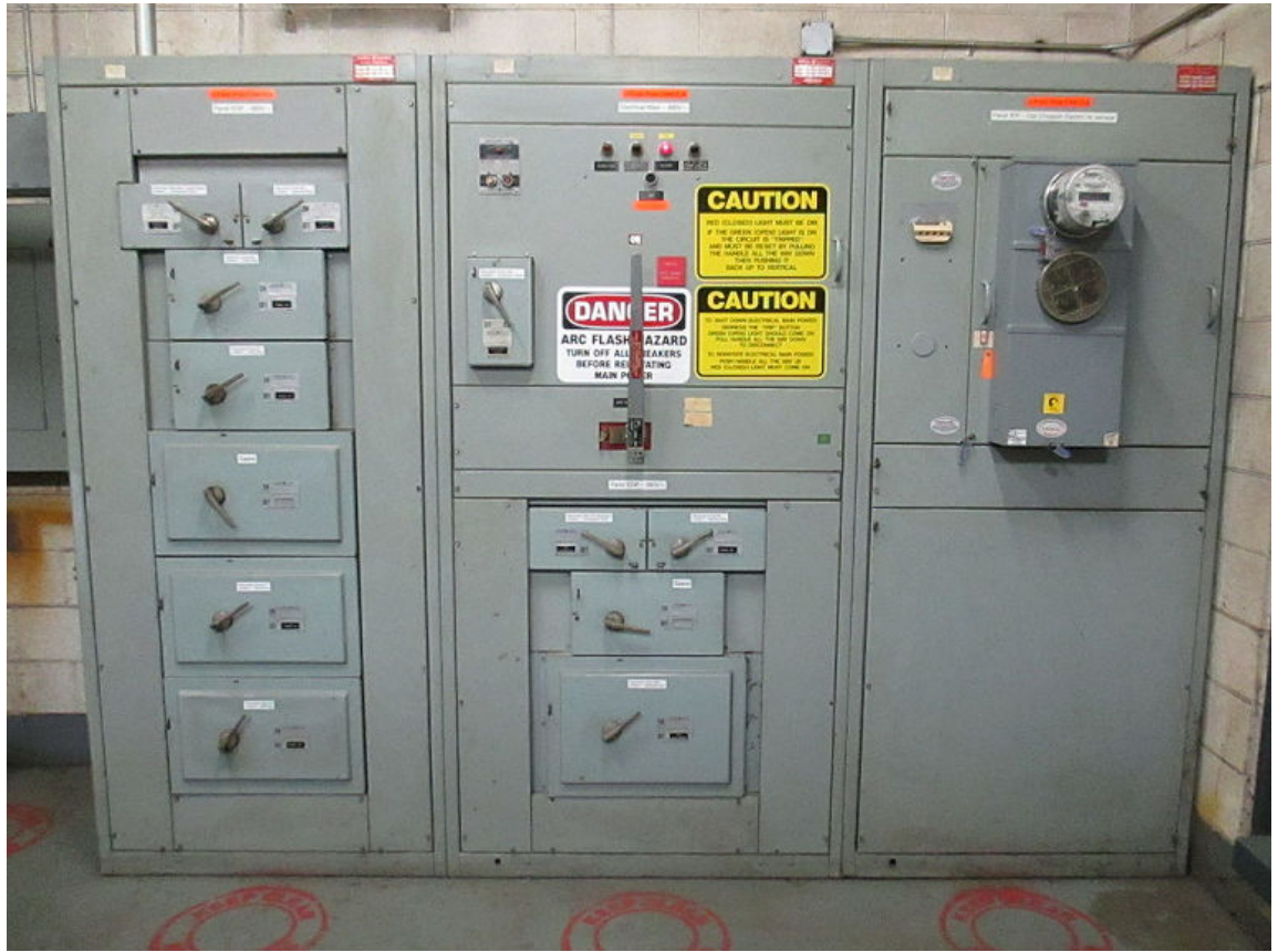
Figure 3–15: The switchgear for an electrical main and its associated distribution should be maintained every few years. (Source: Zaereth/Creative Commons (CC BY-SA 4.0)/ https://commons.wikimedia.org/wiki/File:Electrical_Main_and_distribution_panel_for_480_volt.JPG )
