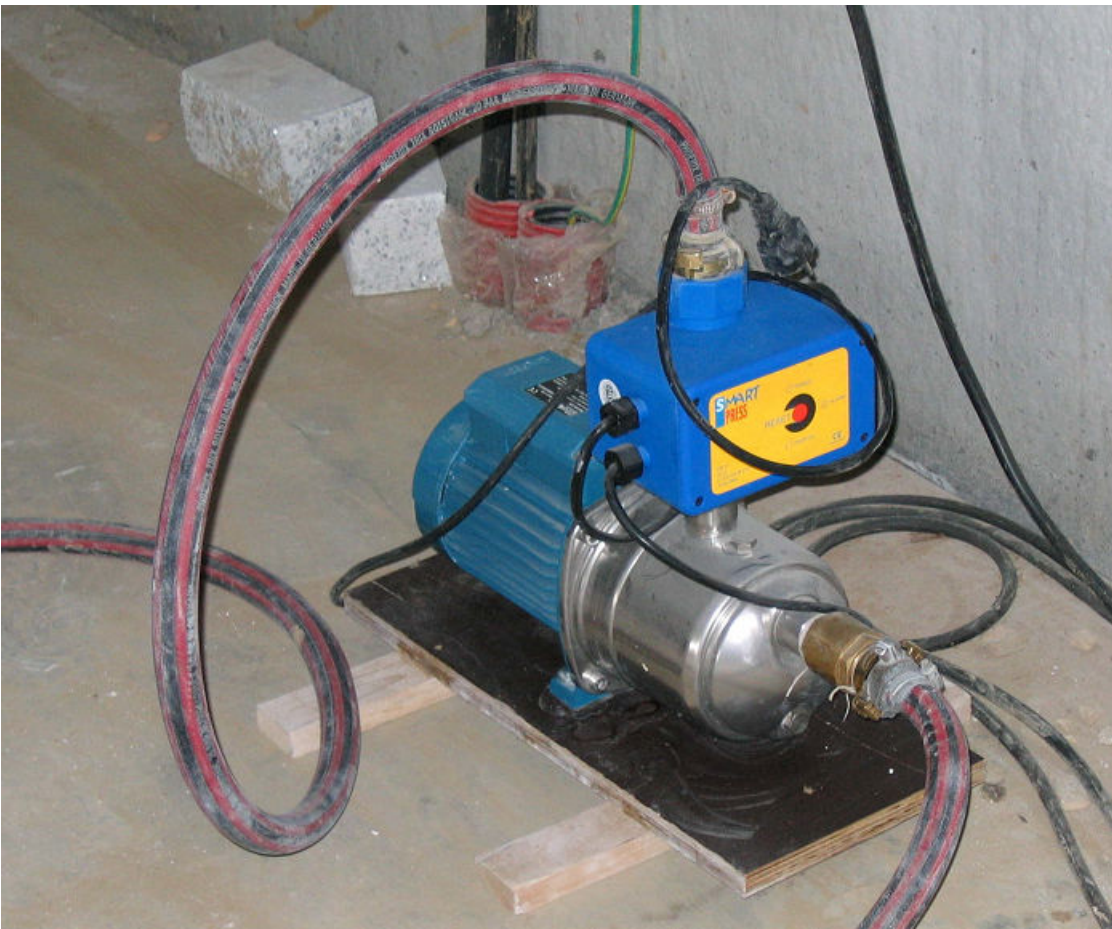
Figure 5-2: A small, electric-powered pump can add pressurization—and therefore increased fluid movement—within the plumbing system. (Source: KVDP/Creative Commons (Public Domain)/ https://commons.wikimedia.org/wiki/File:Jet_pump.jpg )
