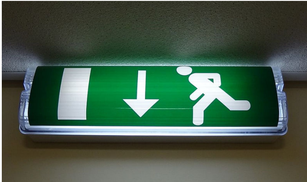
Figure 6–11: An exit sign very visibly tells people where to go to exit the building, especially in the case of an emergency. (Source: KRoock74/Creative Commons (CC BY–SA 3.0)/ https://commons.wikimedia.org/wiki/File:Exit_light_sign.JPG )
