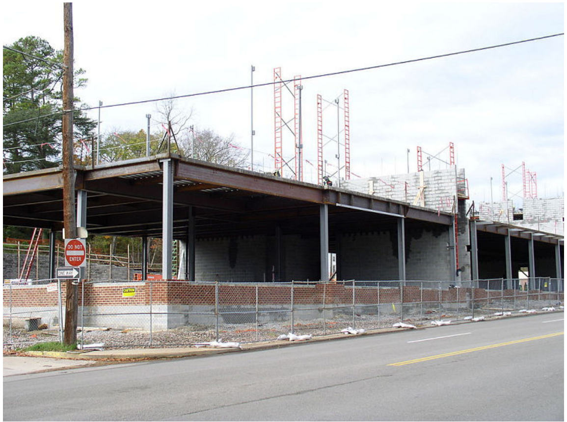
Figure 6–9: The concrete firewalls separating various spaces are clearly visible in a building under construction. (Source: Blahedo/Creative Commons (CC BY-SA 3.0)/ https://commons.wikimedia.org/wiki/File:Firewall_construction_2.JPG )
