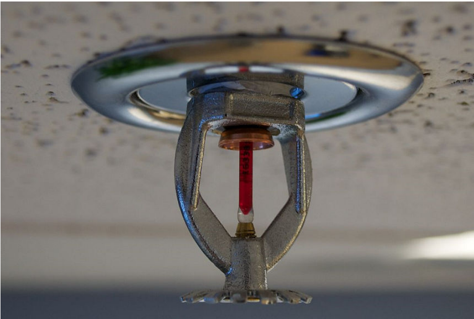
Figure 6–6: A ceiling-mounted sprinkler is part of the larger sprinkler system. (Source: Brandon Leon/Creative Commons (CC BY-SA 2.0)/ https://commons.wikimedia.org/wiki/File:Fire_sprinkler_roof_mount_side_view.jpg )
