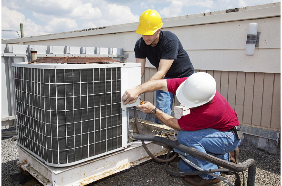
Figure 1-17: HVAC technicians work on an air conditioning unit for a building. (Source: lisafx/iStock/Thinkstock)
