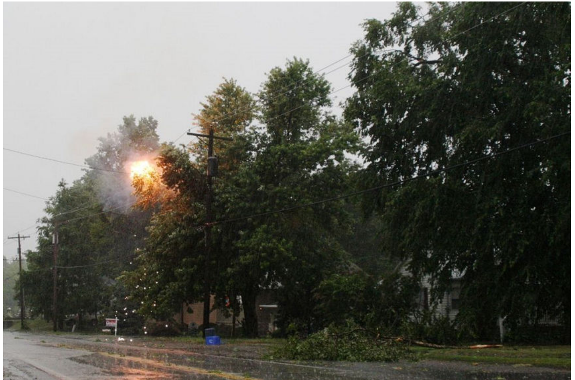
Figure 7–7: Inclement weather brings down tree branches on power lines, causing a utility outage. (Source: Robert Lawton/Creative Commons (CC BY-SA 2.5)/ https://commons.wikimedia.org/wiki/File:Crossed_wires.JPG )
