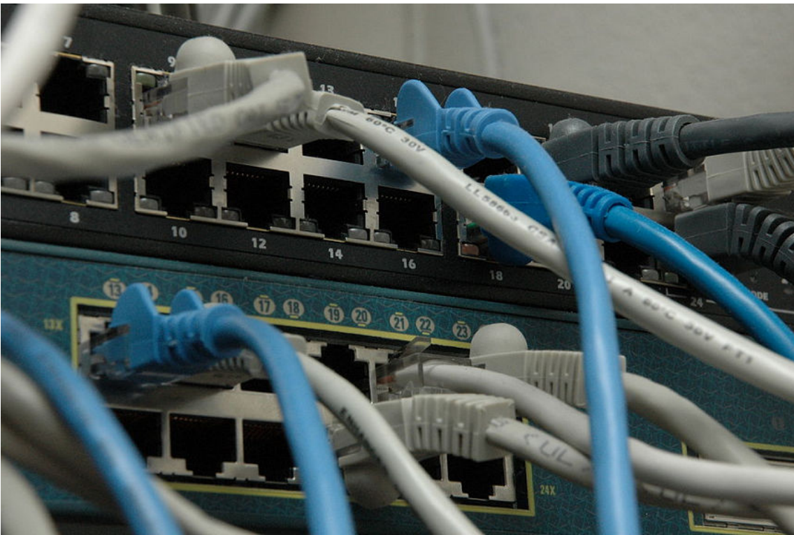
Figure 10–4: Two rack-mounted network switches with connected cables. (Source: ShakataGaNai/ Creative Commons (CC BY-SA 3.0/ https://commons.wikimedia.org/wiki/ File:Network_switches.jpg )
