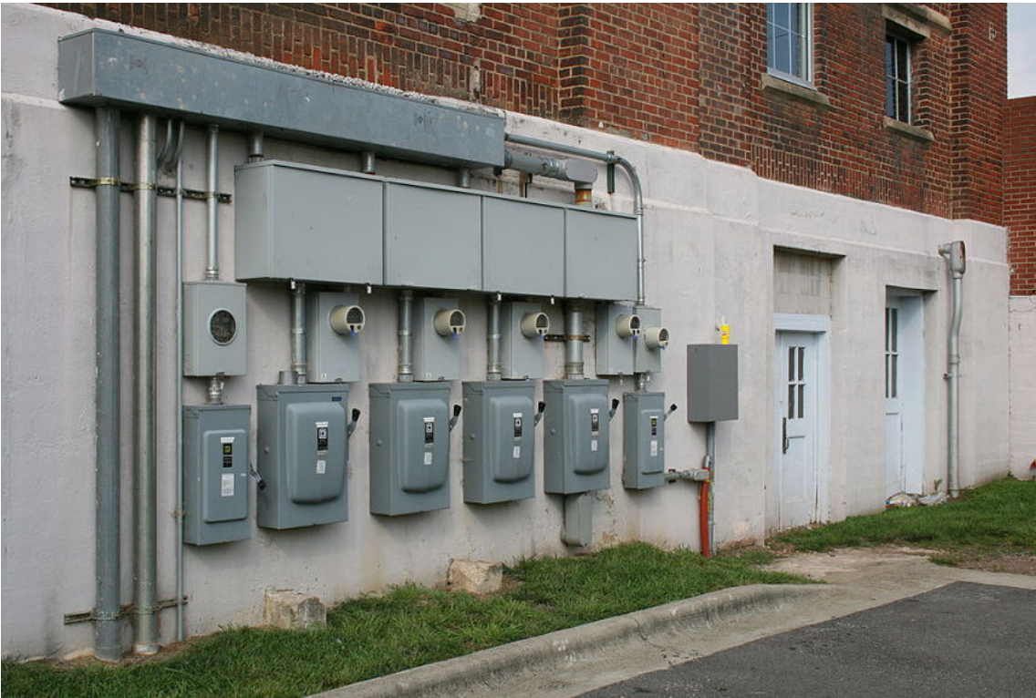
Figure 12-5: Multiple power meters and switches on the exterior of a commercial building. (Source: Ildar Sagdejev/Creative Commons (CC BY-SA 4.0)/ https://commons.wikimedia.org/wiki/File:2008-07-26_Electrical_meters_and_switches_in_Durham.jpg )
