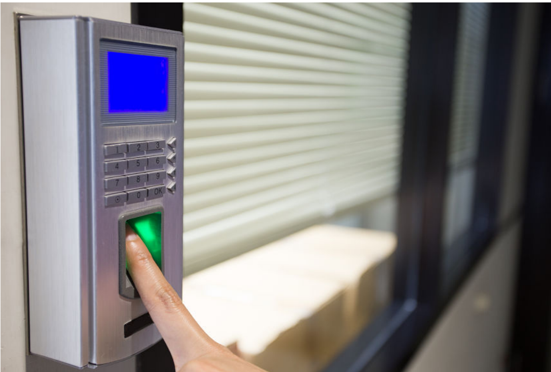
Figure 8–11: A fingerprint scanner allows access to a space to authorized personnel. (Source: Tatom/iStock/Thinkstock)
