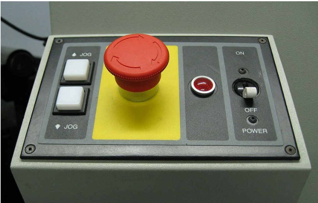
Figure 6–12: An EPO kill switch for a piece of machinery equipment in a laboratory. (Source: Cjp24/Creative Commons (CC BY-SA 3.0)/ https://commons.wikimedia.org/wiki/File:Emergency_stop_button.jpg )
