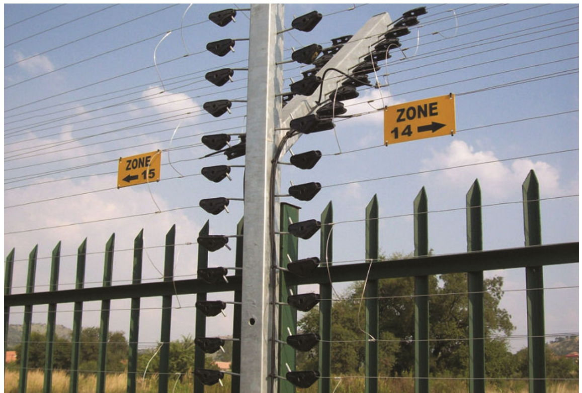
Figure 8-3: A multi-zone electrical fence installed on top of other fencing serving as a physical barrier to entry. (Source: PaktonDale/Creative Commons (CC BY-SA 4.0)/ https://commons.wikimedia.org/wiki/File:Security_Electric_Fence.JPG )
