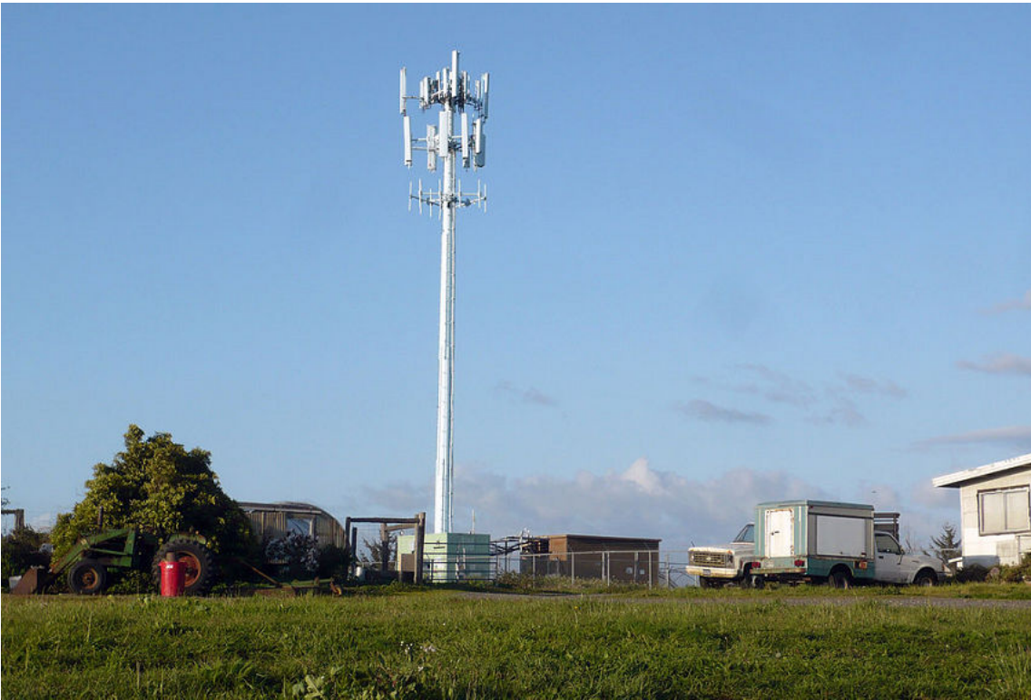
Figure 11-5: A cellular communications tower. (Source: Ellin Beltz/Creative Commons (Public Domain)/ https://commons.wikimedia.org/wiki/File:Cell_TowerTableBluffCA.JPG )
