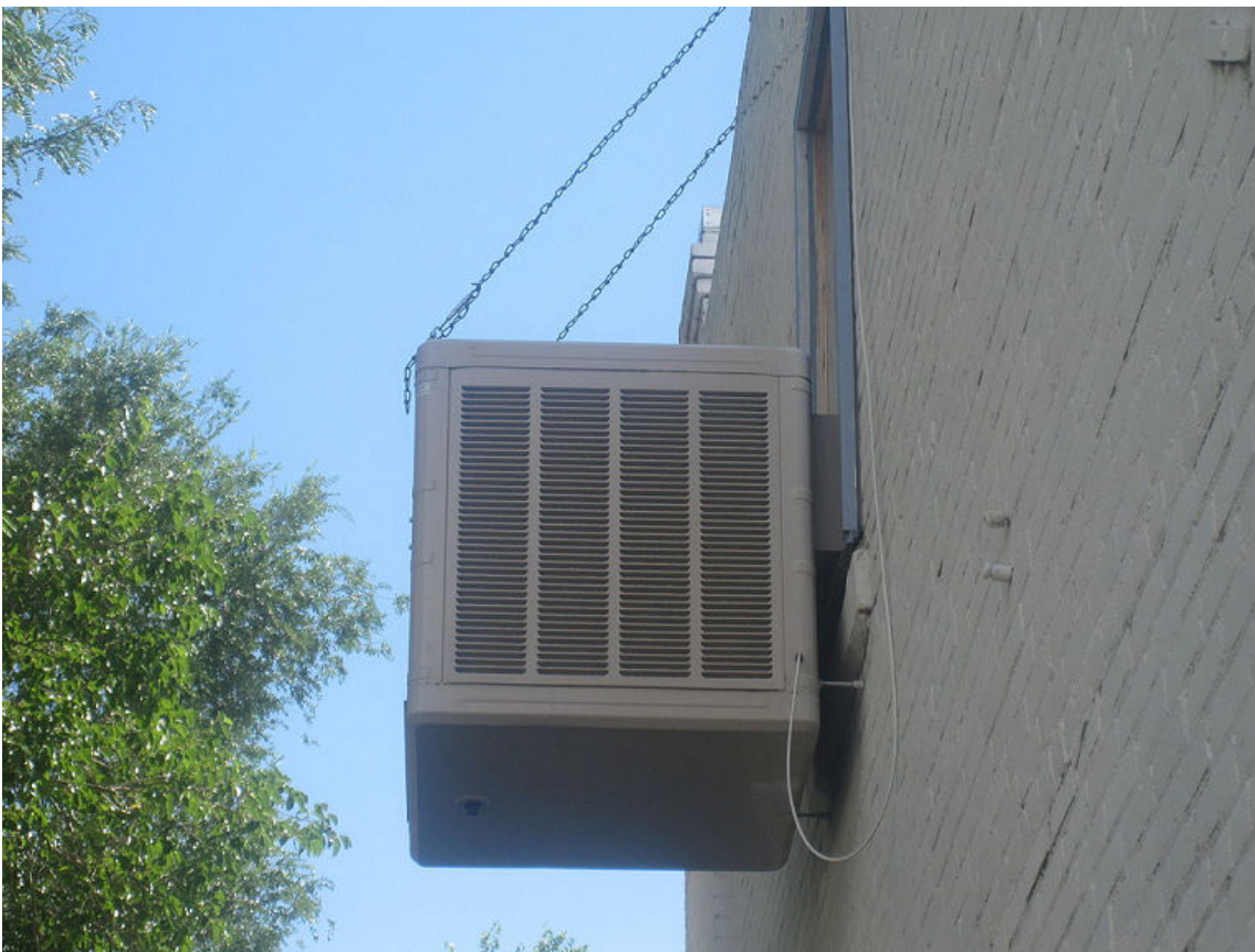
Figure 4-14: An evaporative cooler hangs off the side of the building in Colorado, where drier conditions allow it to be used as a source of cool air. (Source: Billy Hathorn/Creative Commons (CC BY-SA 3.0)/ https://commons.wikimedia.org/wiki/File:Evaporative_cooler,_CO,_IMG_5681.JPG )
