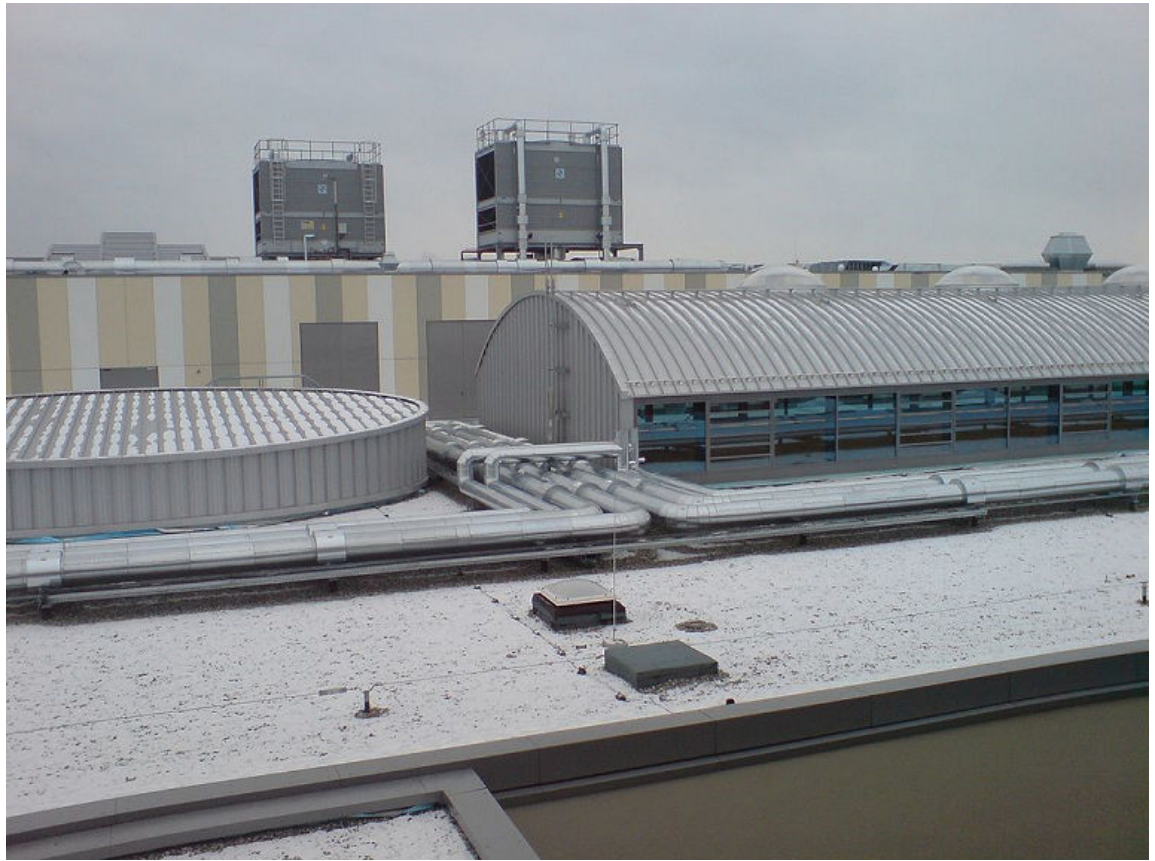
Figure 4–10: HVAC cooling towers on top of a shopping mall remove heat from the facility. (Source: Ingolfson/Creative Commons (Public Domain)/ https://commons.wikimedia.org/wiki/File:Loop_Shopping_Centre_Exterior_1.jpg )
