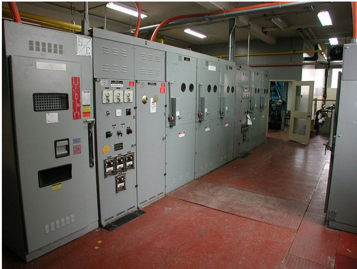
Figure 2–12: A paralleling switchgear in an MCO facility. (Source: P199/Creative Commons (Public Domain)/ https://commons.wikimedia.org/wiki/File:Electrical_switchgear.JPG )
