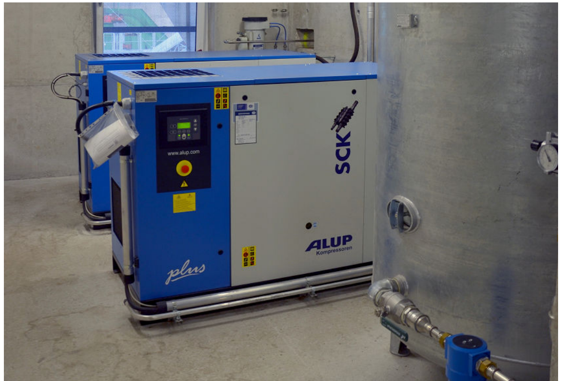
Figure 5–5: An air compressor station creates and delivers pressurized air for use in a power plant. (Source: Sensenschmied/Creative Commons (CC BY–SA 3.0)/ https://commons.wikimedia.org/wiki/File:Kompressorstation_mit_Druckluftspeicher.jpg )
