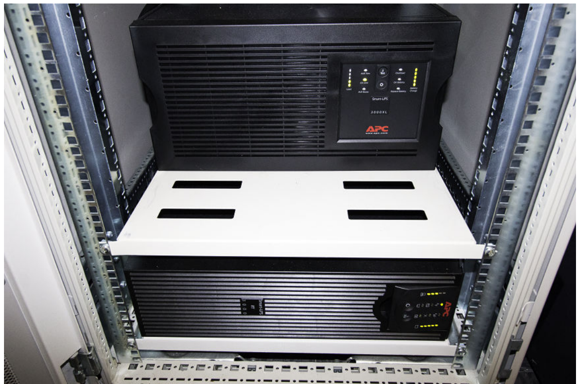
Figure 2–13: A UPS on server racks in a small-scale data center. (Source: Logical Operations for NCMCO)
