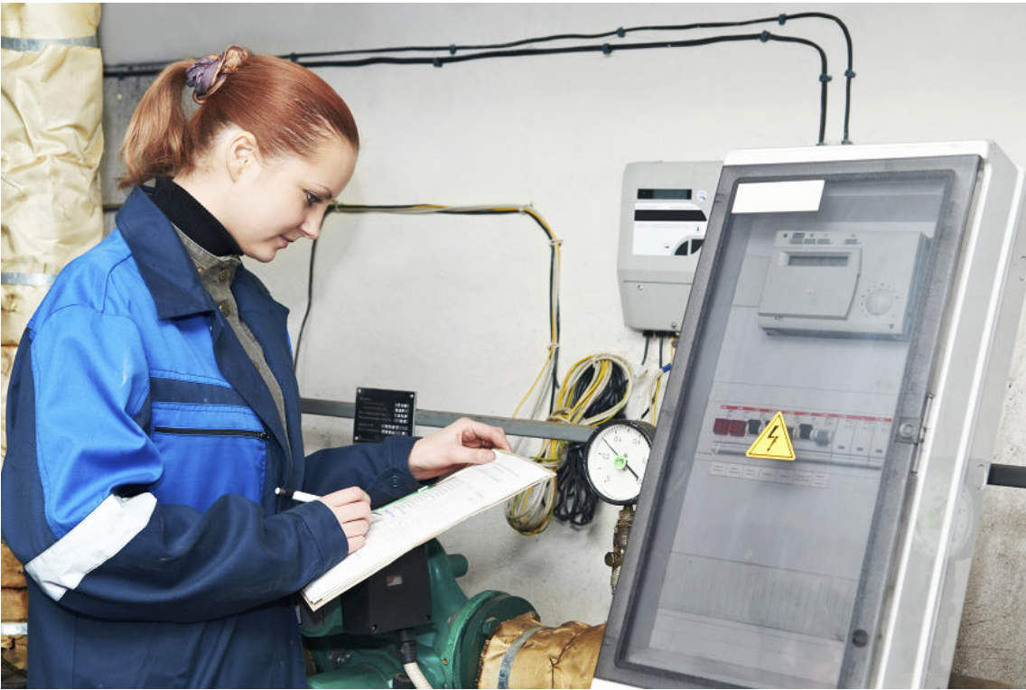
Figure 5–9: An MCO technician performs rounds and readings for the components in a boiler room. (Source: Dmitry Kalinovsky/iStock/Thinkstock)
