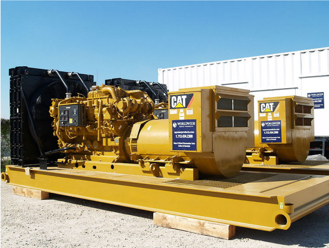
Figure 3-16: Any generator sets onsite, whether backup or primary, should be exercised on a monthly basis. (Source: StcudorPrewoP/Creative Commons (CC BY-SA 3.0)/ https://commons.wikimedia.org/wiki/File:Caterpillar_3512C_Generator_Set.JPG )
