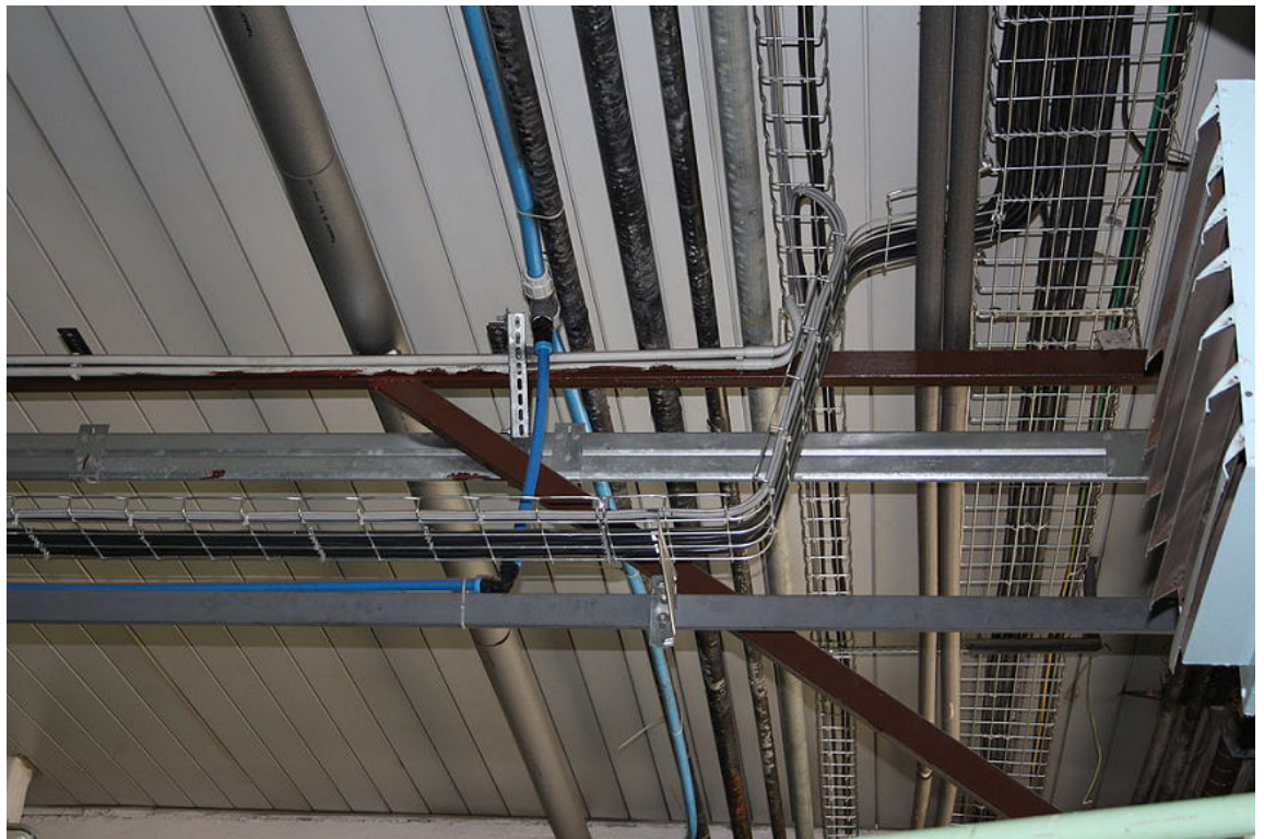
Figure 9–8: Overhead cable trays run cables throughout a space. (Source: Leotard/Creative Commons (Public Domain)/ https://commons.wikimedia.org/wiki/File:Wire_cable_tray02.jpg )
