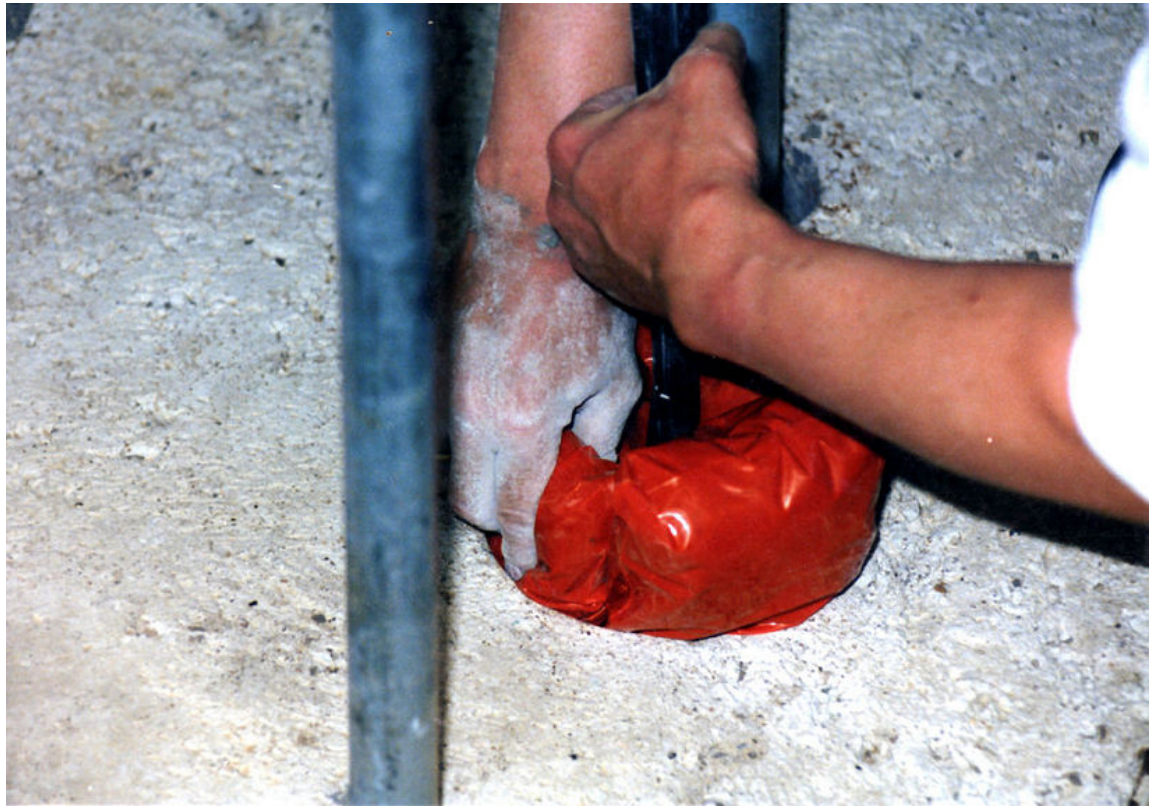
Figure 6–10: A firestop pillow is installed in a penetration in a concrete slab to provide fire protection. (Source: Achim Hering/Creative Commons (CC BY 3.0)/ https://commons.wikimedia.org/wiki/File:Pillowinst.jpg )
