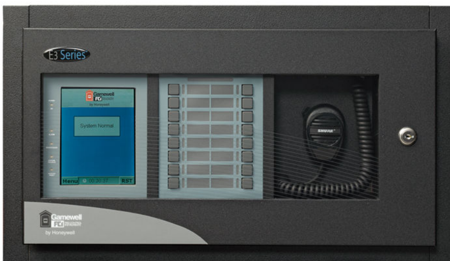
Figure 12–10: A console for a mass notification system displays a notification that the system is in a normal state. (Source: Gamewell-FCI (Bcarl)/ https://commons.wikimedia.org/wiki/File:Local_Operating_Console_(LOC).jpg )
