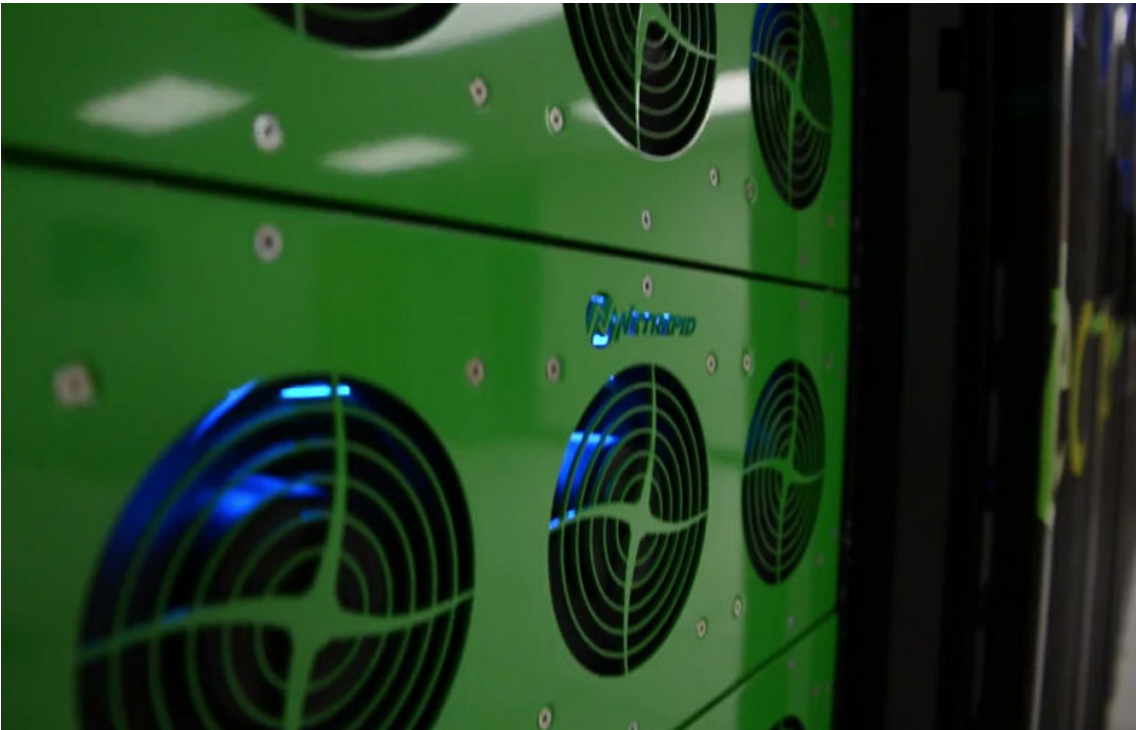
Figure 9–3: The fans on a server rack are used to moderate the temperatures of the servers on the rack. (Source: Annagen, LLC dba Netrepid/Creative Commons (CC BY-SA 3.0)/ https://commons.wikimedia.org/wiki/File:Colocation_Cooling_Rack.png )
