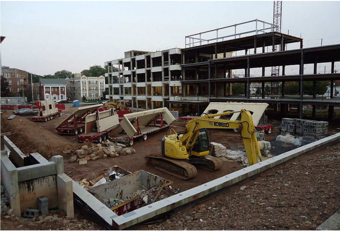
Figure 13–8: The construction of a new building would have to comply with the unified standards of the International Building Code. (Source: Tomwsulcer/Creative Commons (Public Domain)/ https://commons.wikimedia.org/wiki/File:Summit_NJ_Construction_Site_DeForest_Avenue.jpg )
