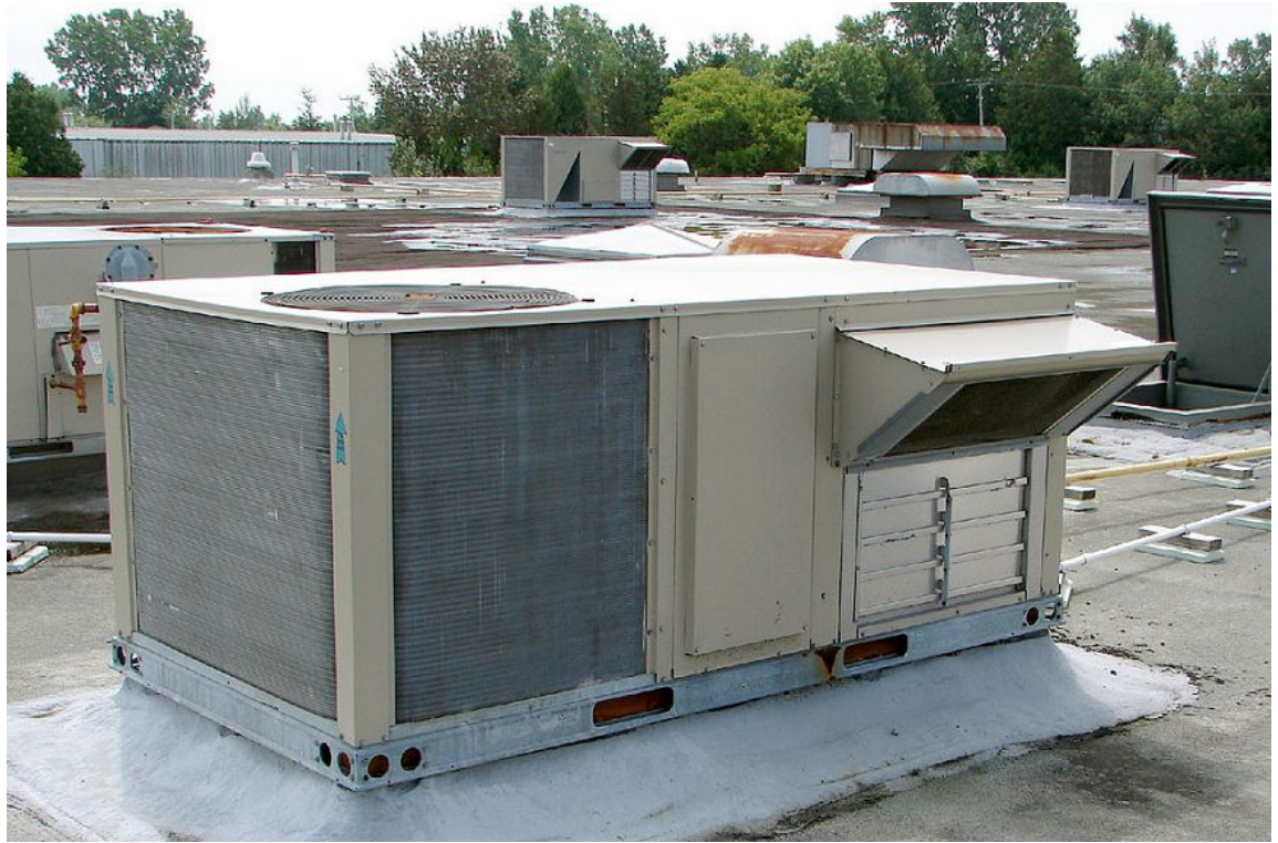
Figure 4–16: A rooftop air handling unit. (Source: P199/Creative Commons (Public Domain)/ https://commons.wikimedia.org/wiki/File:Rooftop_Packaged_Units.JPG )
