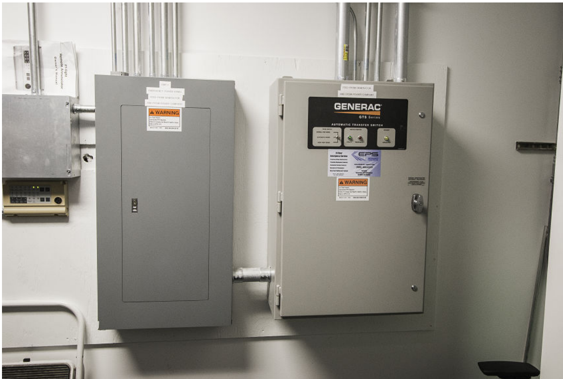
Figure 3–4: An automatic transfer switch connected to the main breaker box. (Source: Logical Operations for NCMCO)
