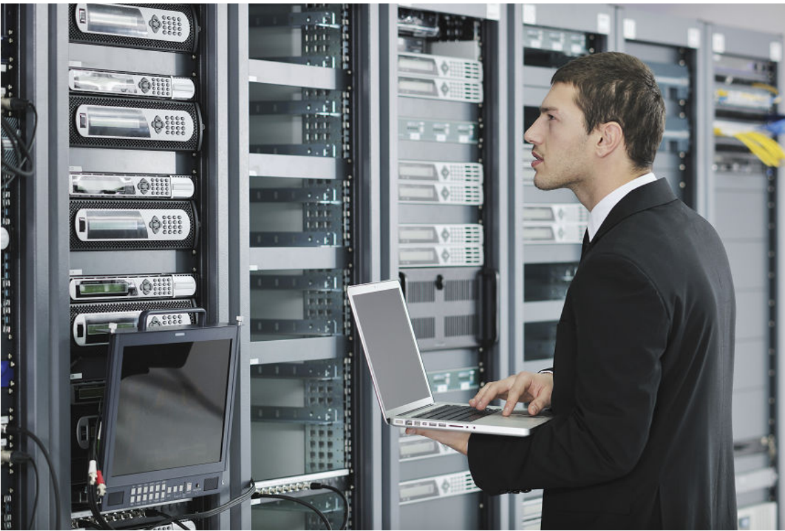
Figure 1-18: A network technician inspects the server stacks in a data center. (Source: .shock/iStock/Thinkstock)
