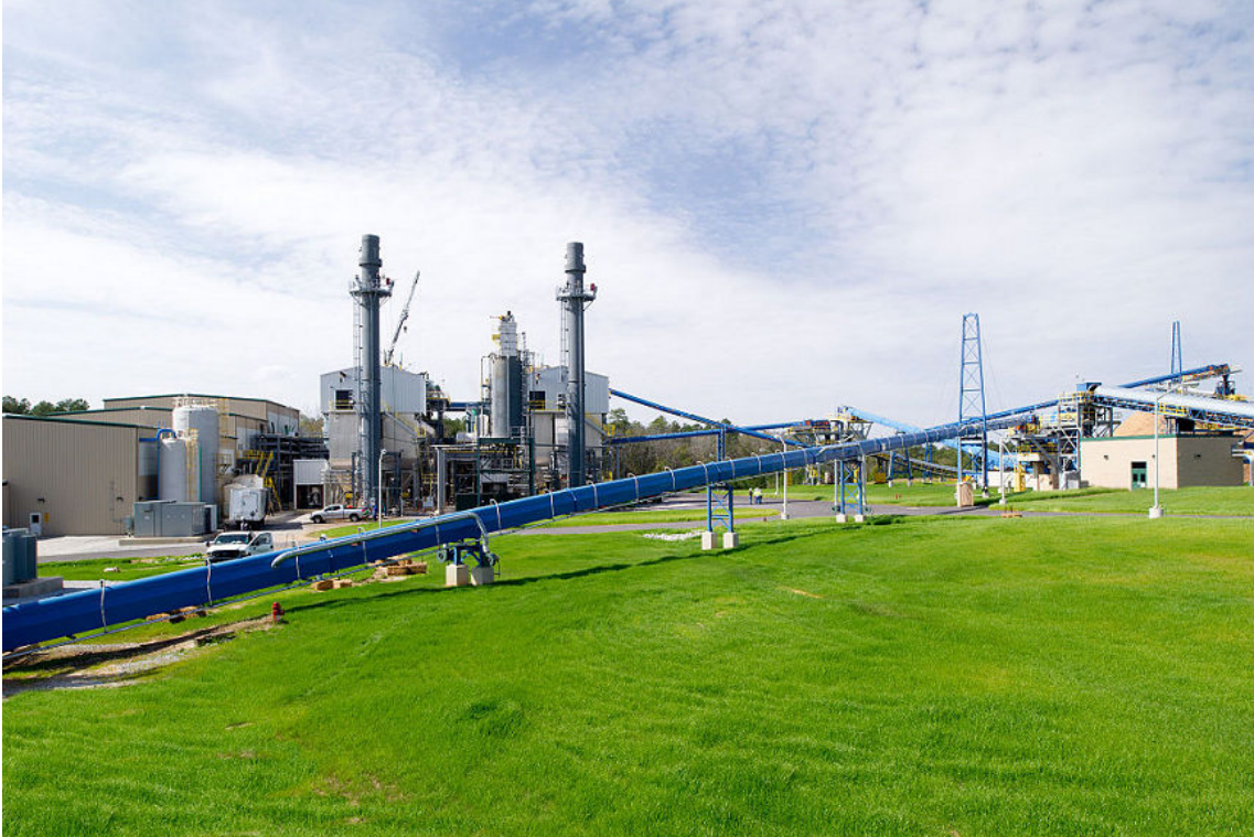
Figure 2–19: The biomass plant at the Savannah River Site in South Carolina burns forest residue to provide power to the rest of the campus, which produces nuclear materials for the U.S. Department of Energy. (Source: United States Department of Energy/Creative Commons (Public Domain)/ https://commons.wikimedia.org/wiki/File:Biomass_being_processed_at_the_Savannah_River_Site_(7609895484).jpg )
