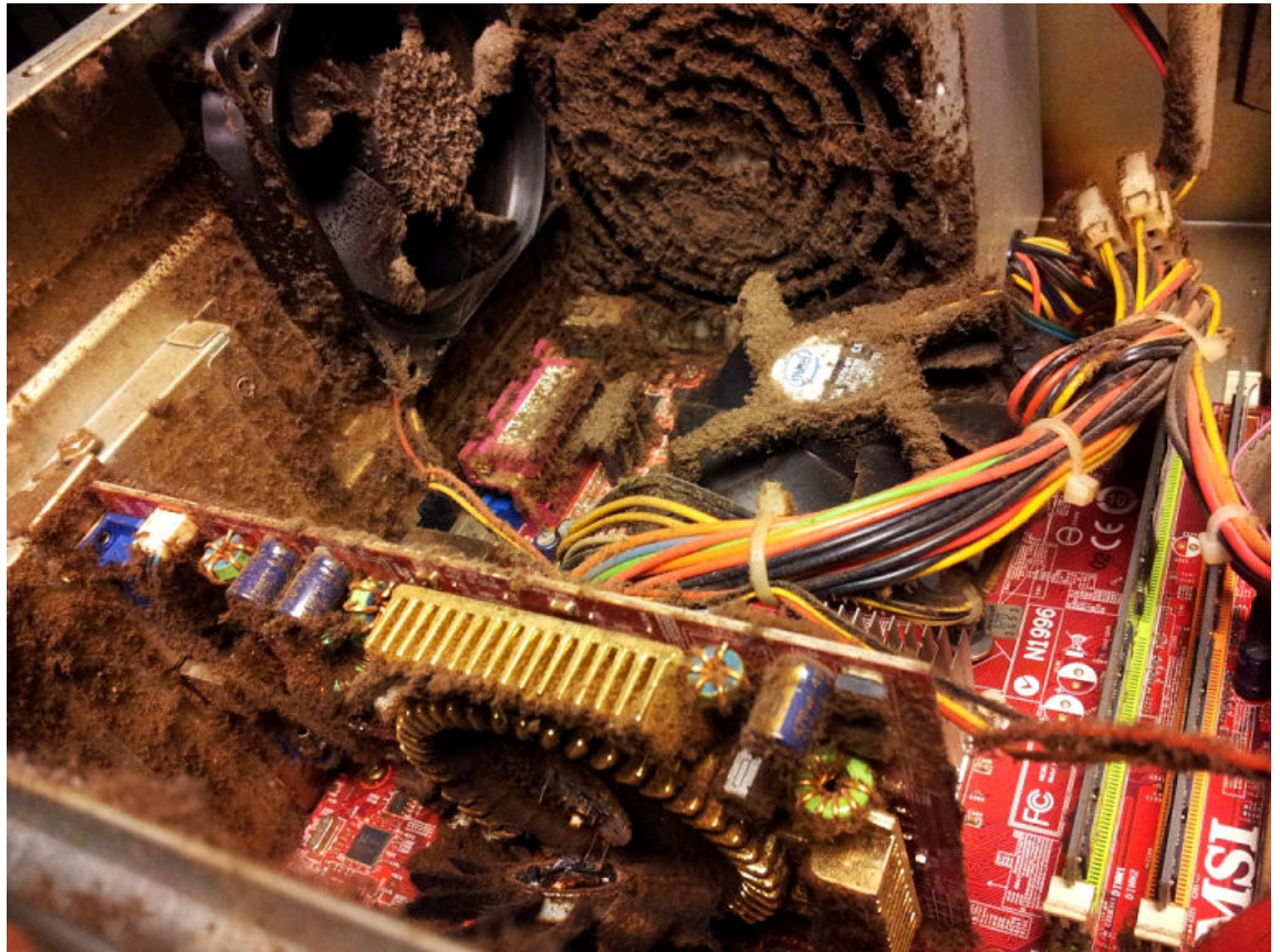
Figure 9-4: Dust has built up inside of a computer that has gone far too long without cleaning, and has led to some component failures. (Source: Arvutistuudio/Creative Commons (CC BY-SA 4.0)/ https://commons.wikimedia.org/wiki/File:Dusty-dirty_PC.jpg )
